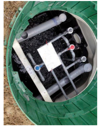
Air lines and recirculation valves are shown in the Fusion's aeration chamber.
