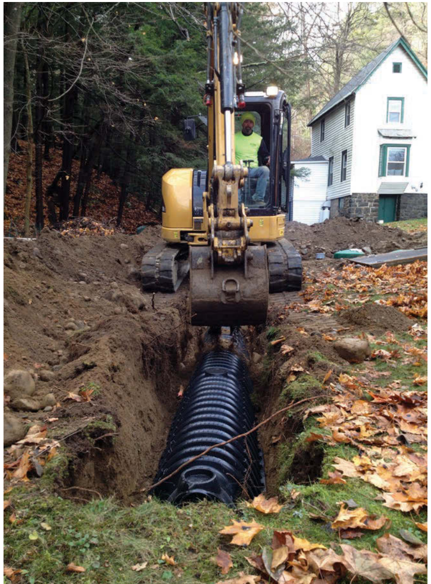
BELOW: Lack of space forces operator Brian Ramos from Stone Installations to dig and backfill trenches with the excavator straddled over them. The trenches hold Arc 24 chambers from Infiltrator Systems.
