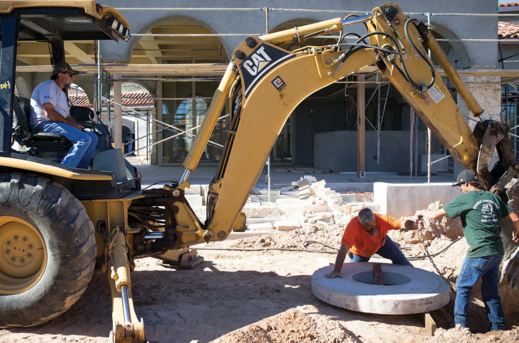
From left, Tim Bottorff, Jim Ralls and J.R. Bottorff use a Cat backhoe to place a riser lid over a water tank at an Arizona home.
