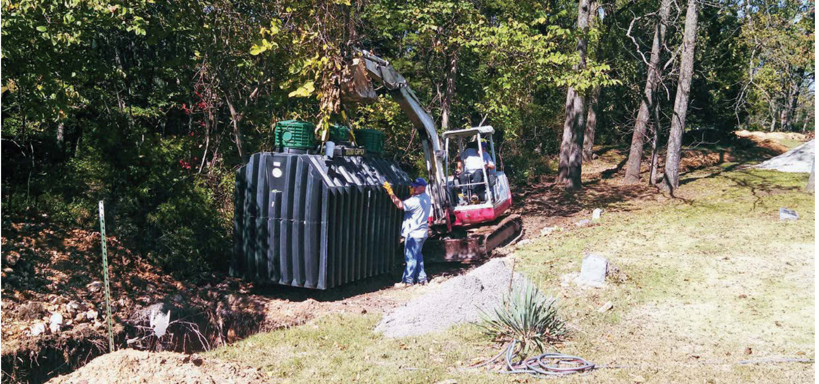
ABOVE: Ben Maness, left, and Kevin Rouse, on the excavator, maneuver the Jet ATU tank into position at Log Providence Missionary Baptist Church in Missouri. Beyond the trees is a sinkhole, and a few feet away are graves.
