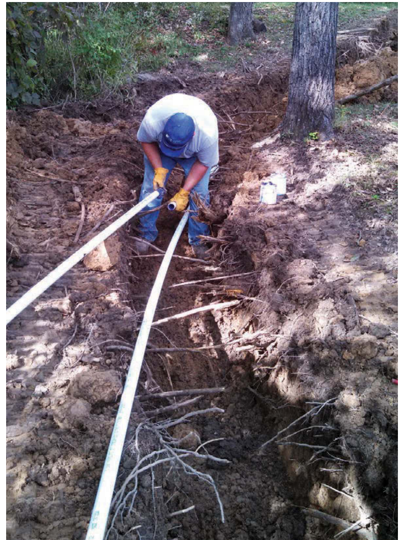
BELOW: Ben Maness assembles 1 1/4-inch pipe to form the dosing and return lines between the Infiltrator dosing tank and the drip irrigation field.
