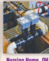
Nursing Home, OH 2 Salcor 3G UV Units in Series with an Activated Sludge Plant. Replaces Chlorination
