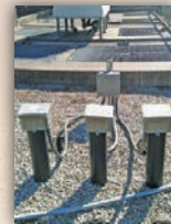
Elementary School, MO 3 Salcor 3G UV Units in a Parallel Array
