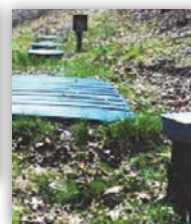
Mud River Project, WV Over 100 Salcor 3G UV Units Installed with ANUA Peat Filters
