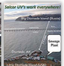
Sewage Plant, AK Little Diomed Island Salcor 3G UV Unit with Lifewater Engineering
