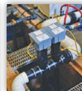
Nursing Home, OH 2 Salcor 3G UV Units in Series with an Activated Sludge Plant. Replaces Chlorination
