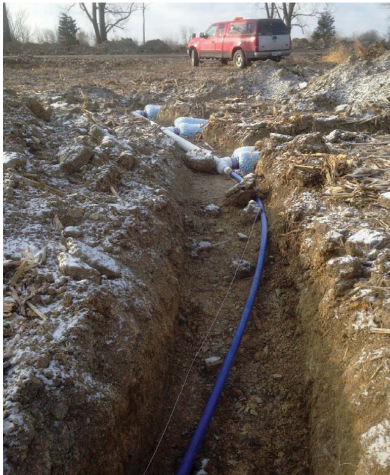
A 2-inch pipe brings water from the MBR to the absorption field where it transitions to the 4-inch pipe that feeds EZflow laterals. Notice that pipes are also paired with a tracer wire to make locating easier.
