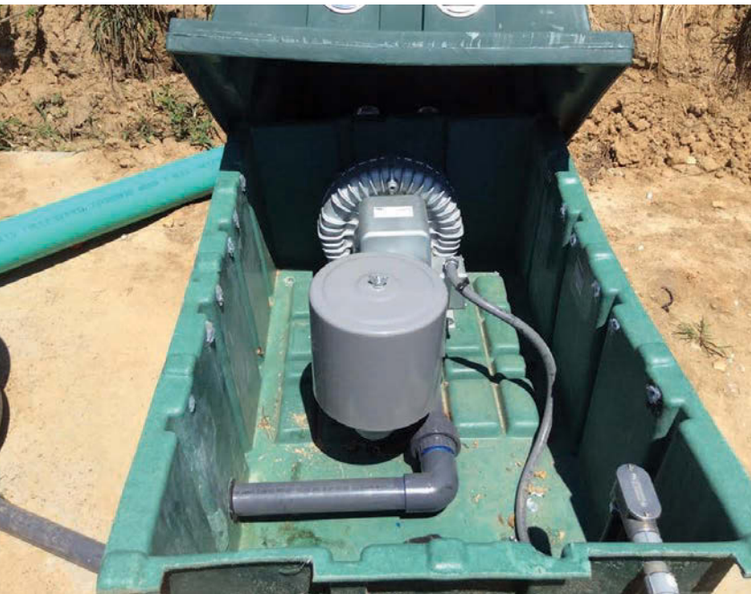
The Bio-Microbics FAST system includes this Gast Regenair blower model R6150J-2 cfm open 60/50 Hz: 215. The chamber holding the unit is vented with a single 6-inch pipe.
