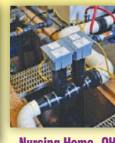
Nursing Home, OH 2 Salcor 3G UV Units in Series with an Activated Sludge Plant. Replaces Chlorination
