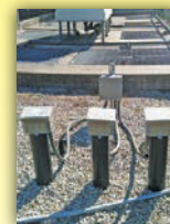
Elementary School, MO 3 Salcor 3G UV Units (Parallel Array) in Extended Aeration
