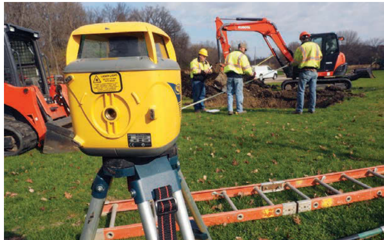
A Spectra HR 500 laser level is shown in the foreground as Tom Wirtzfeld, Tim Barry and Nick Simonsen use Kubota equipment during a system installation at McCullough Park in Shieldsville, Minnesota.
