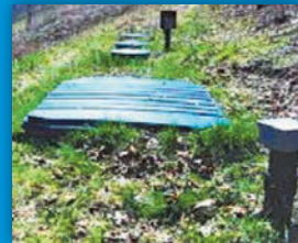
MUD RIVER PROJECT, WV 100+ UV Units w/ANUA Peat Filters
