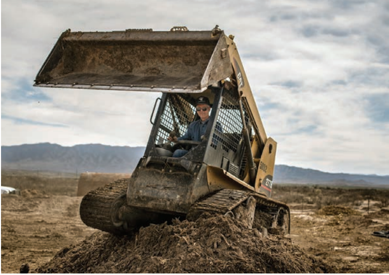
Ensor uses a Caterpillar 277B multi-terrain loader to move waste and wood chips at his composting facility.
