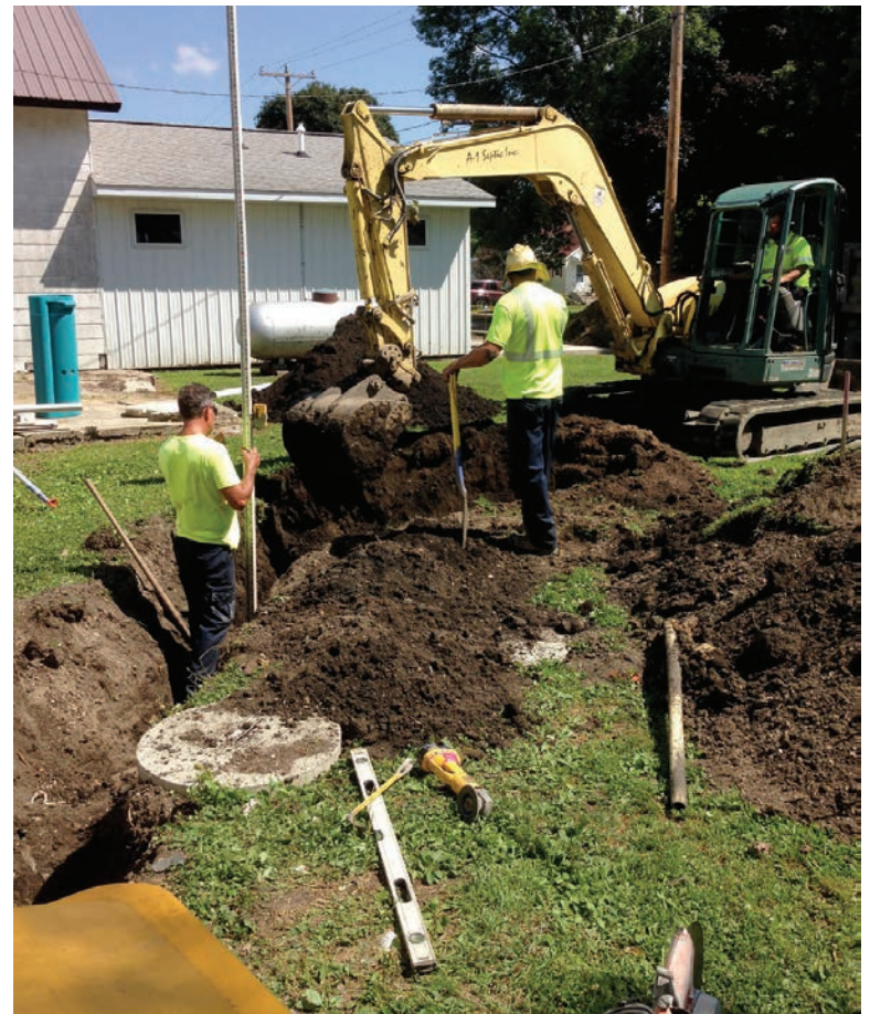
Rick Amundson (left), Eric Morf (center) and Colby Nichols (right) of North Iowa Septic Solutions cut a trench for some of the piping in the community wastewater system for Woden, Iowa. They’re using the company’s Yanmar excavator for the job.
