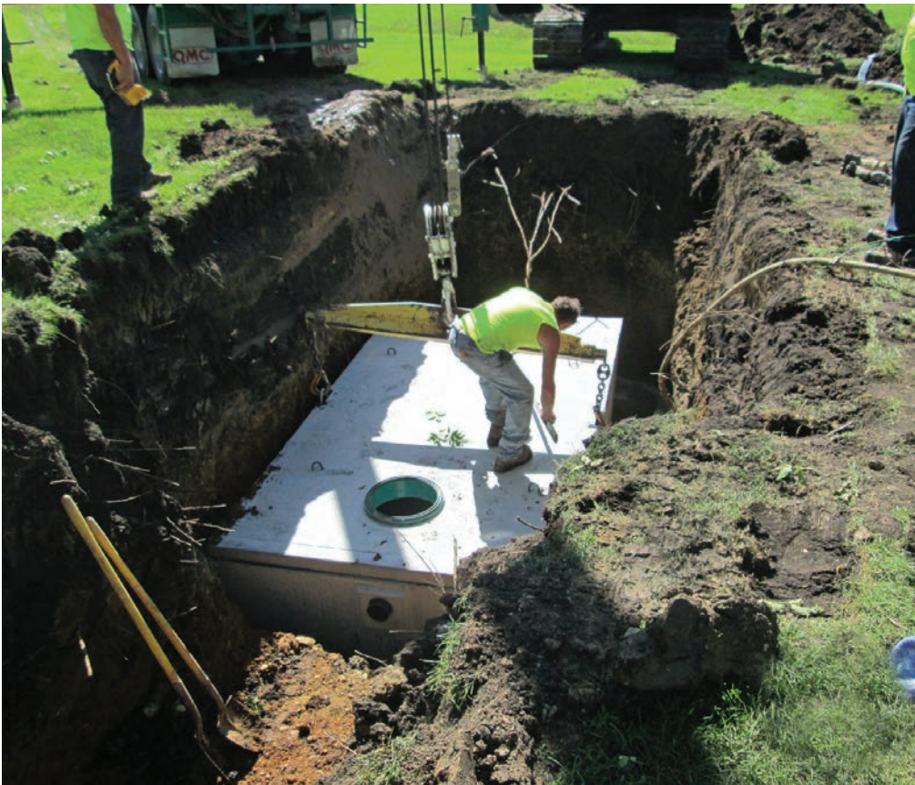
Technician Rick Amundson from North Iowa Septic Solutions sets one of the Wieser Precast Steps tanks in Woden, Iowa. The small community now uses a combined system consisting of septic tanks and a lagoon.
