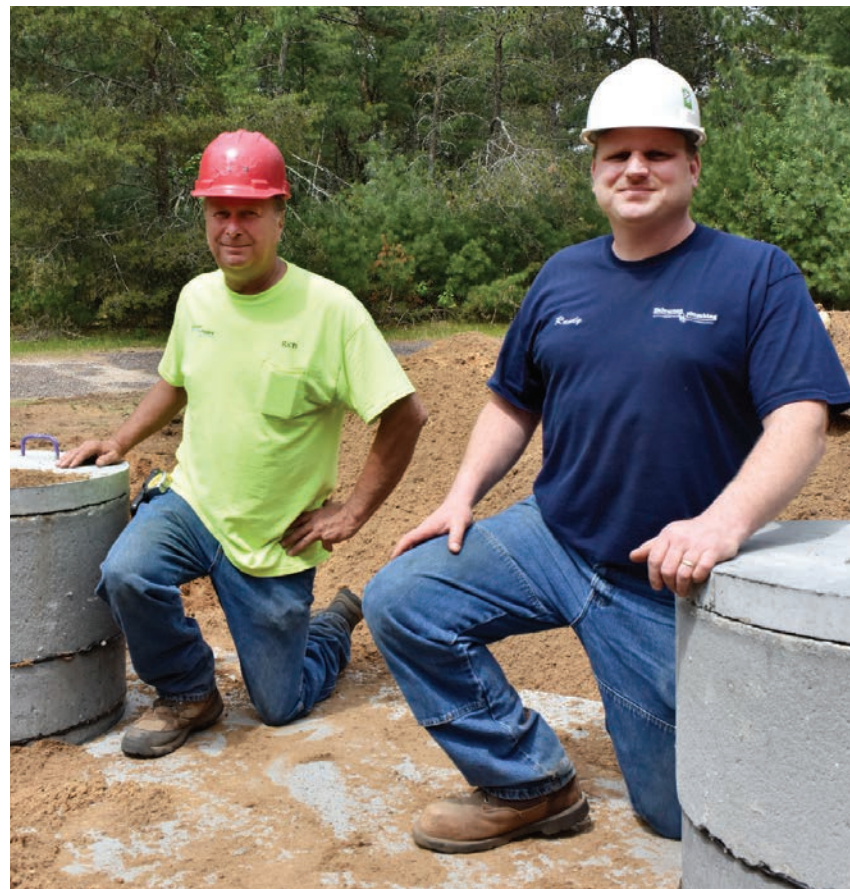
BELOW: Former owner and current employee Rich Halverson, left, and new owner Randy Dolesy, of Halverson Plumbing.
