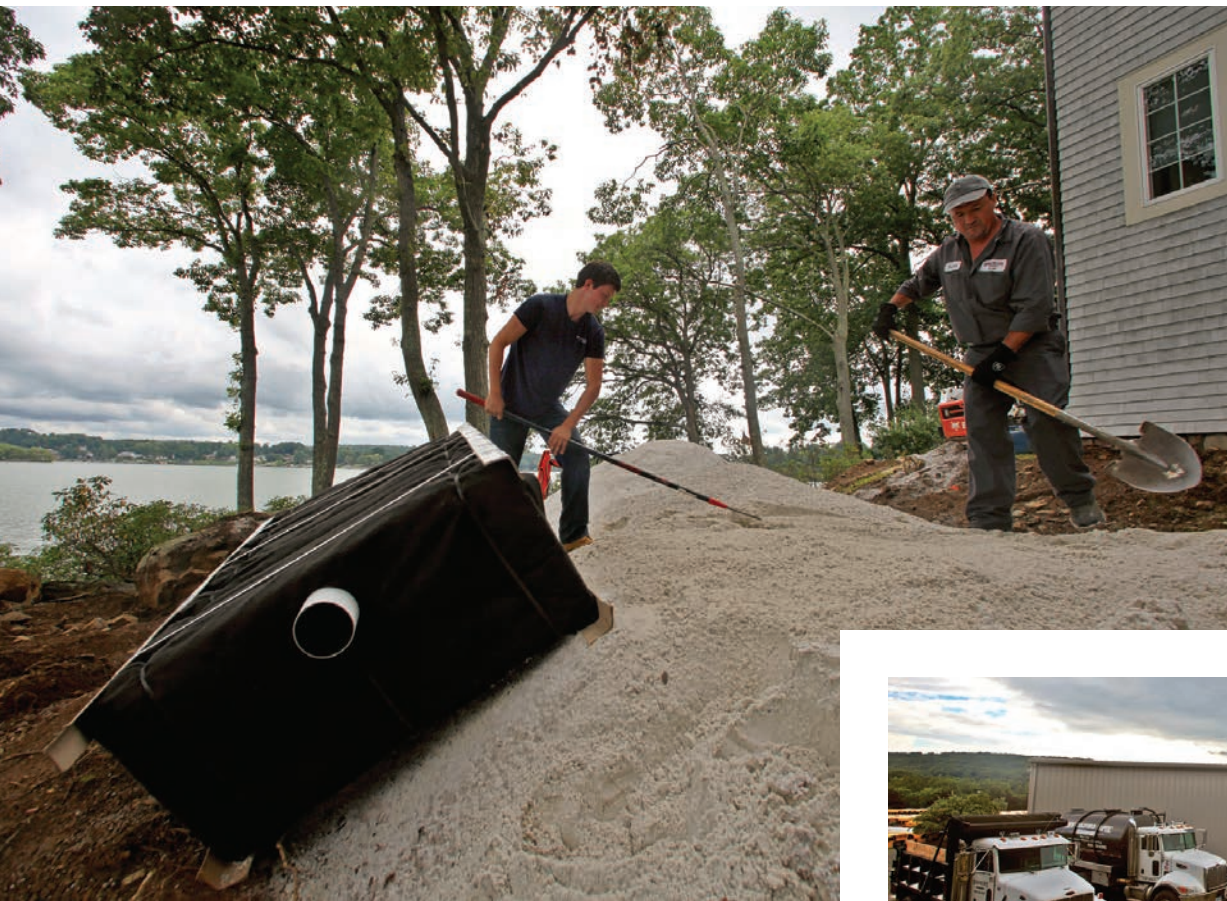
LEFT: Cameron Cunningham, left, and Roberto Alvarez, of New Milford Septic, work on a bed of select fill that will hold a row of 10 Eljen Corp. Mantis units.
