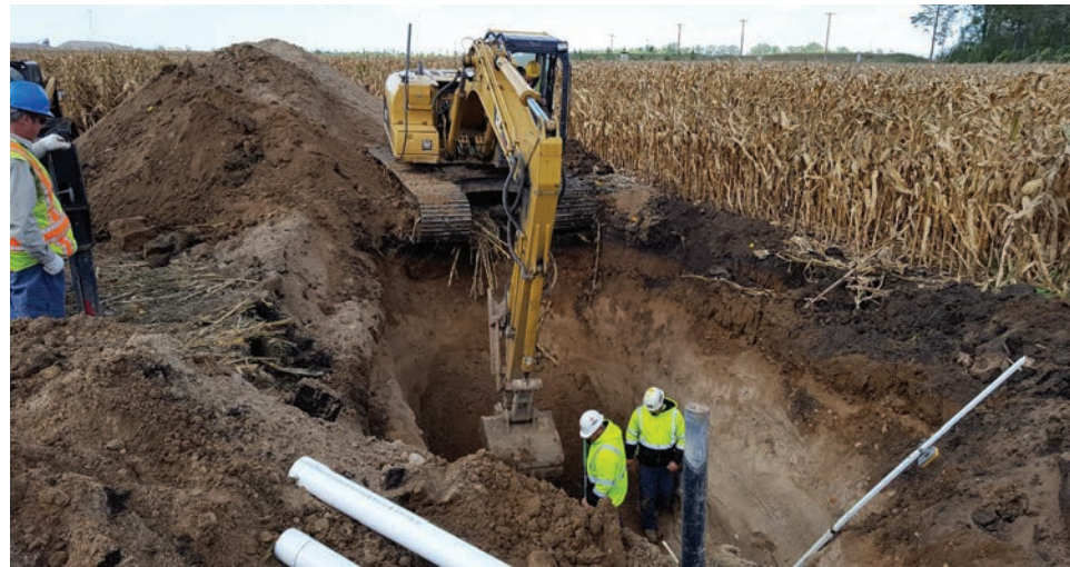
These workers are complying with hard hat and safety vest requirements, but are working with no shoring protection directly beneath a 50,000-pound excavator. (Photos courtesy of the Washington On-Site Sewage Association)
