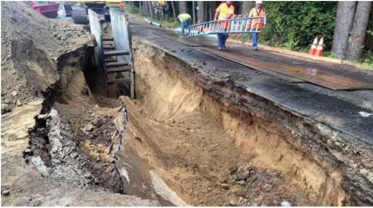
▲ This 21-foot-deep excavation collapsed before shoring could be installed.
