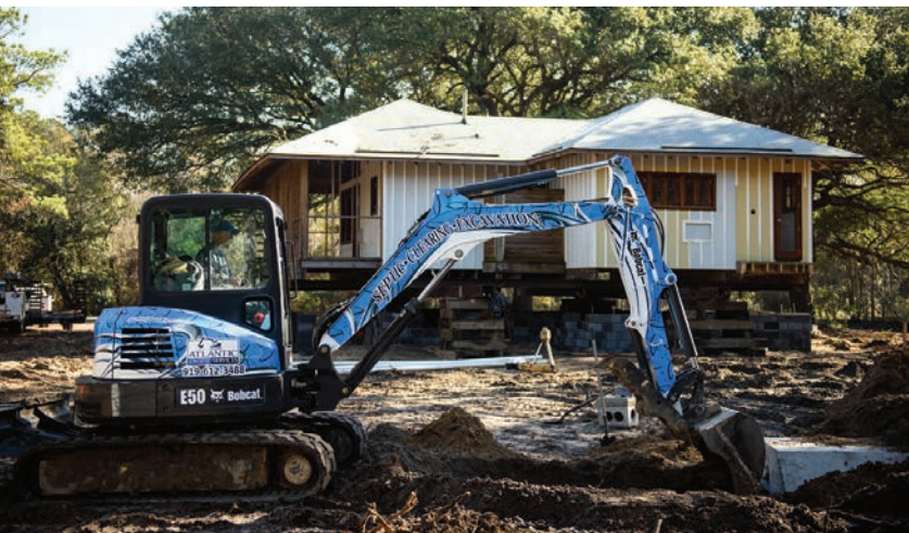
Jesus Cheluca works a Bobcat E50 excavator to dig a trench for a septic system in Sneads Ferry, North Carolina.
