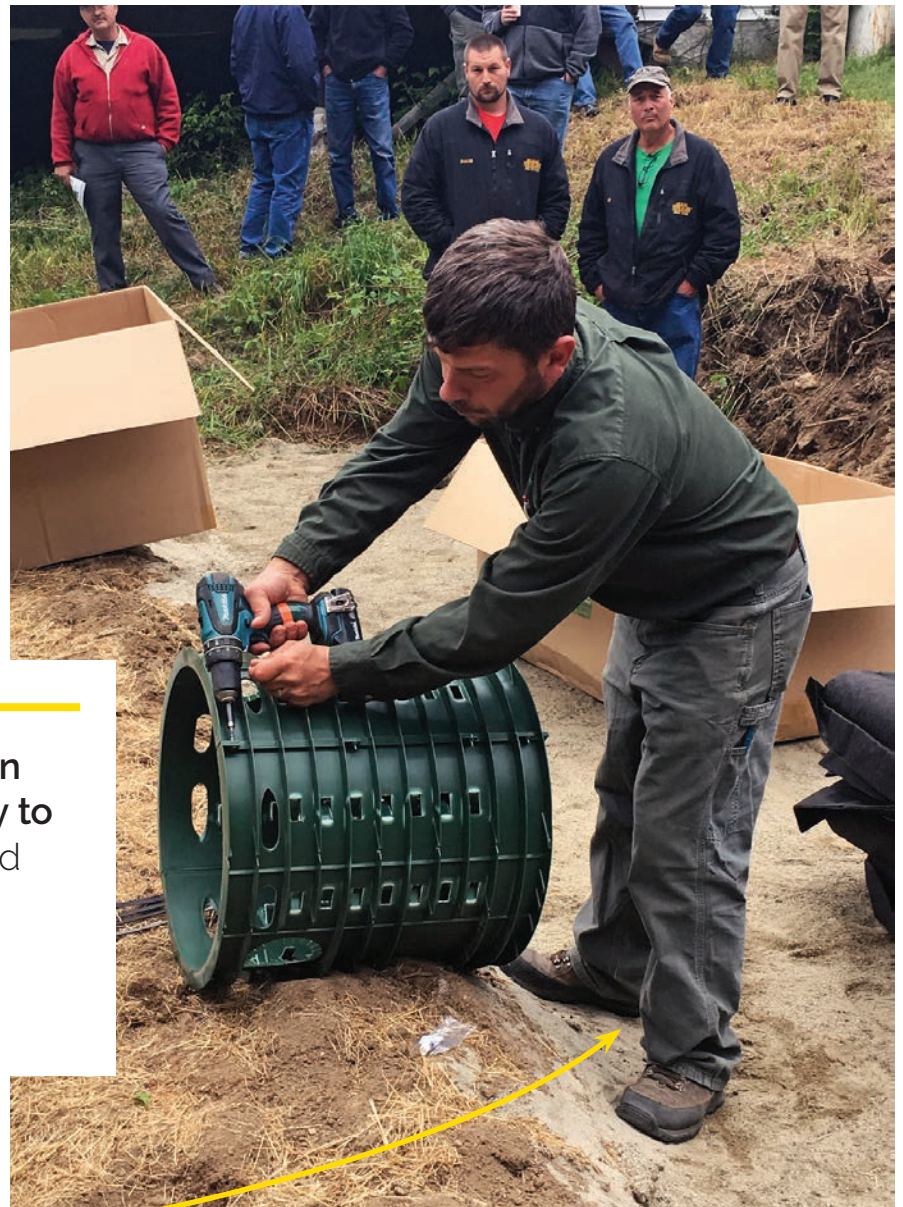
▲ Mike Carbonneau, owner of Connecticut Valley Design in Littleton, New Hampshire, demonstrates where to screw together the two halves of the EnviroFin distribution unit. (Courtesy of Presby Environmental)
