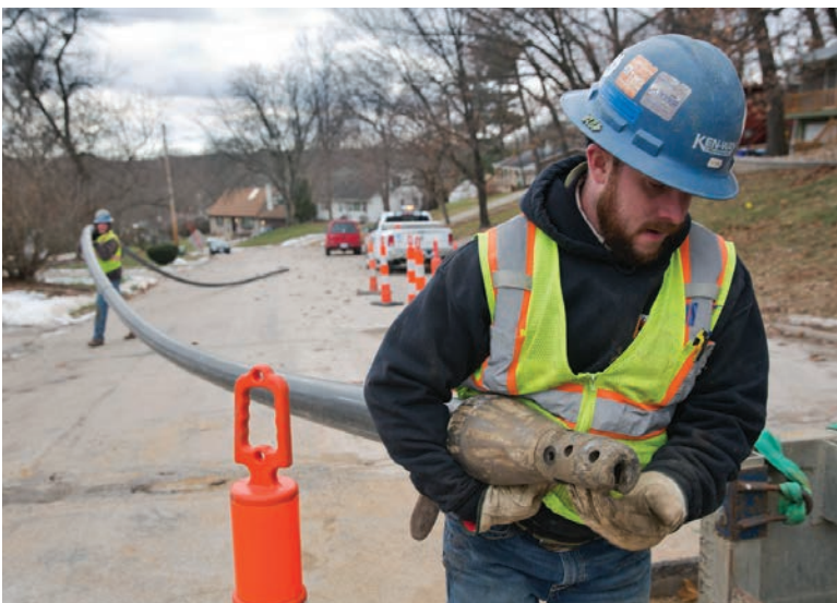
▼ Kyle Jacobson carries a 4-inch HammerHead Quick Grip Burst Head attached to SDR-17 pipe in preparation for drawing it through a damaged pipe.
