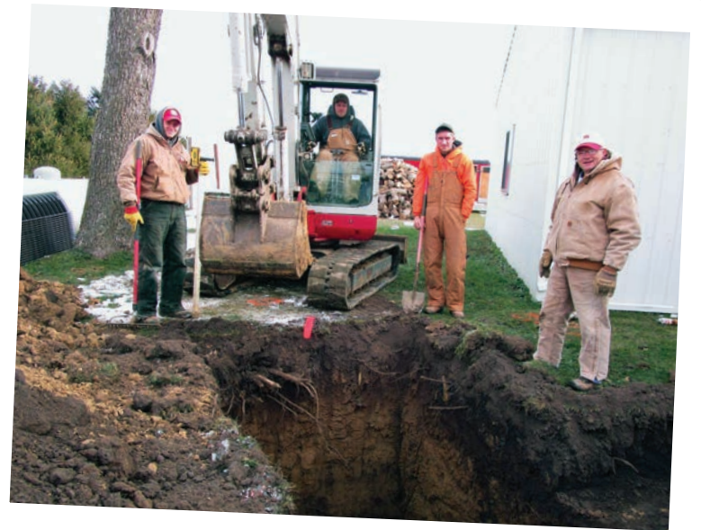
▲ A crew of volunteers including, from left, Nathan Williams, Zach Brown, Caleb DeHamer and Dennis Sullivan installs a new septic system for a family in northwest Illinois. (Photo by Claudia Loucks)
