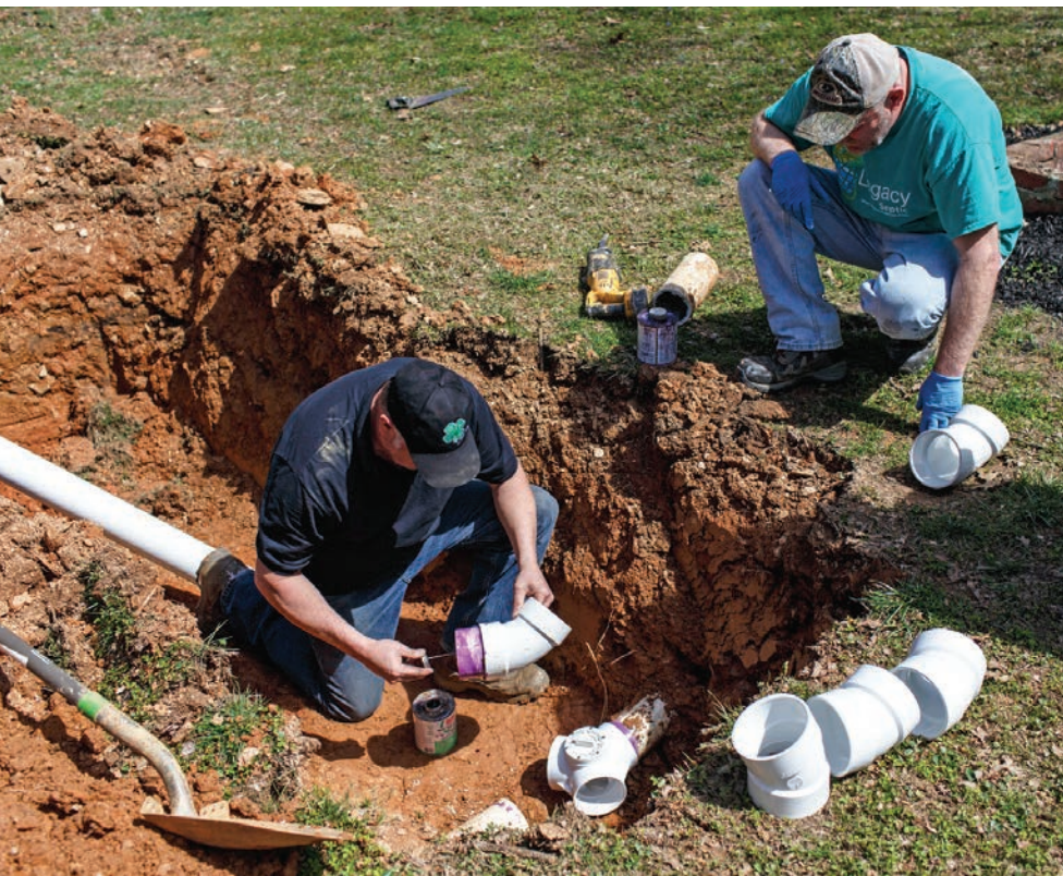
▲ As a worker looks on, George Schooley installs a valve in a trench system. (James Robinson photo)
