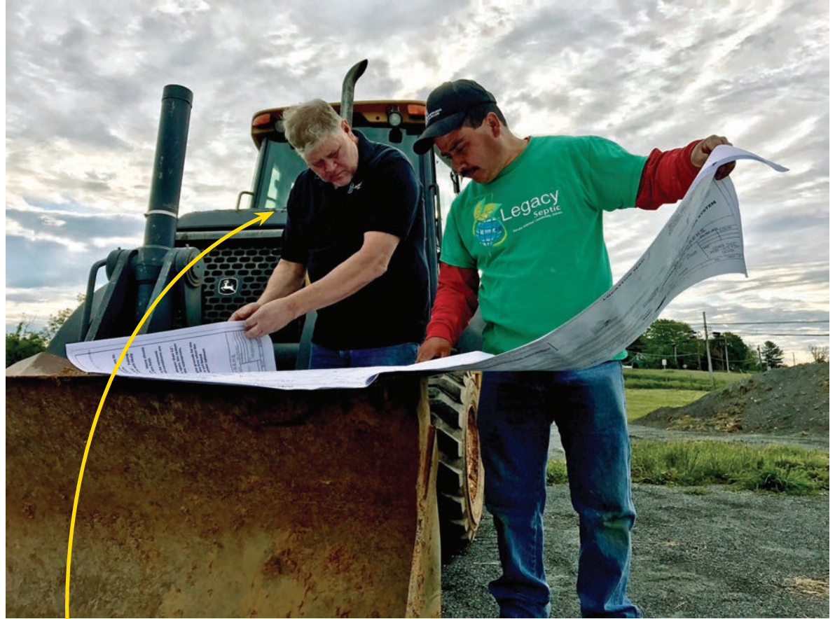
▲ George Schooley, left, reviews onsite system plans with technician Ernesto Sanchez Fernando. (Jenny Walsh photo)
