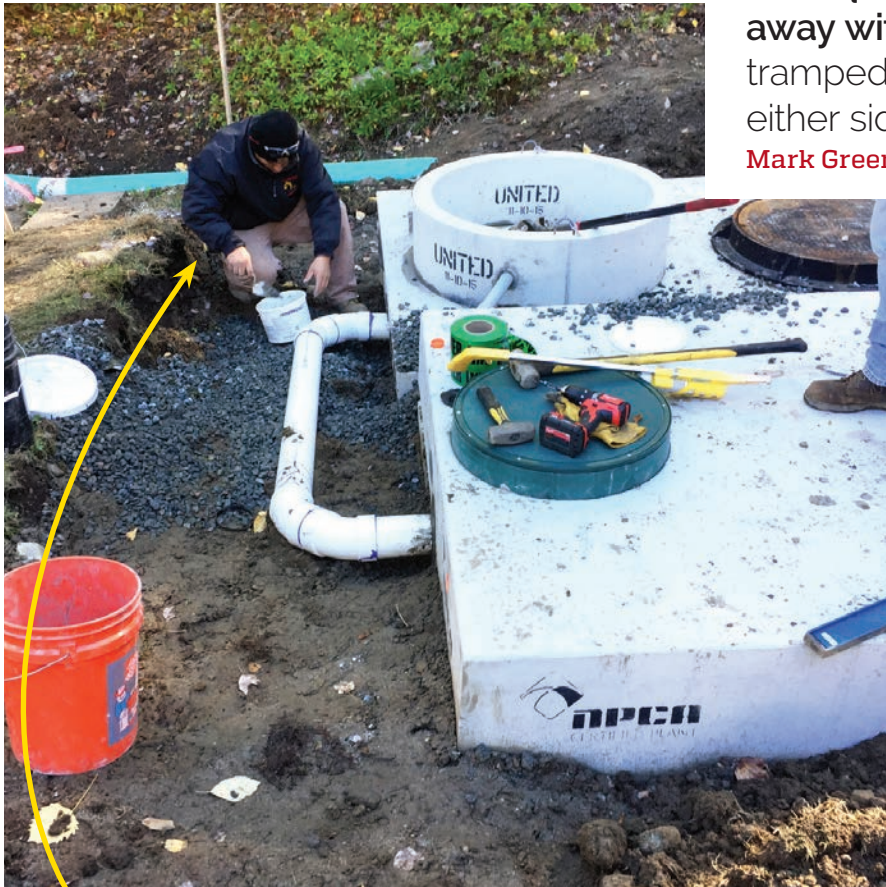
▲ Jovany Sandoval from Green Construction Management mixes mortar in front of the 4-inch pipe connecting the United Concrete Products Low-boy septic tank to the dose tank.
