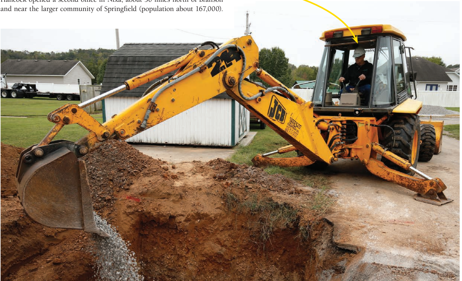
▼ Jon Hancock operates a JCB North America backhoe while preparing a hole for a new septic tank.
