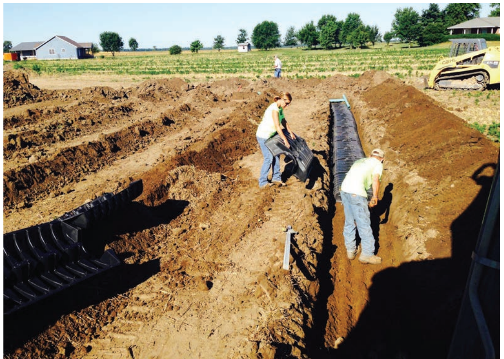
▲ Lisa Black and Kelly Kaeck install Infiltrator Water Technologies Quick4 Plus chambers in a drainfield. A Mustang-Gehl CTL85 skid-steer is used to backfill.
