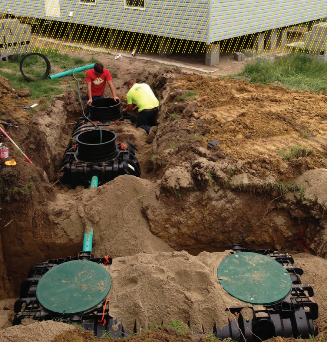
▲ Summer helper Cole Kirchoff, left, and Colby Black install Infiltrator Water Technologies septic and pump tanks for a new mobile home.
