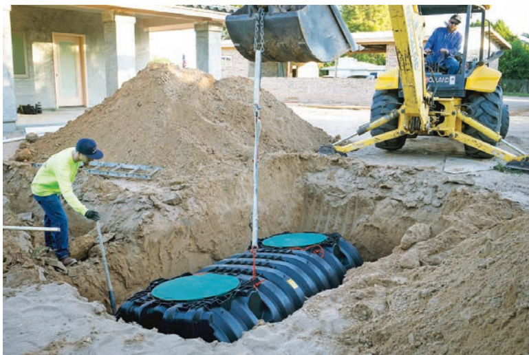
▲ Jereme Tuggle lowers an Infiltrator Water Technologies IM-1060 tank while David Tuggle maneuvers it into place.
