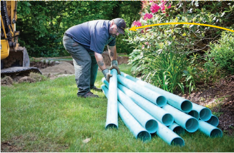
◀ John Sgambato delivers a load of pipe for a septic system install.
