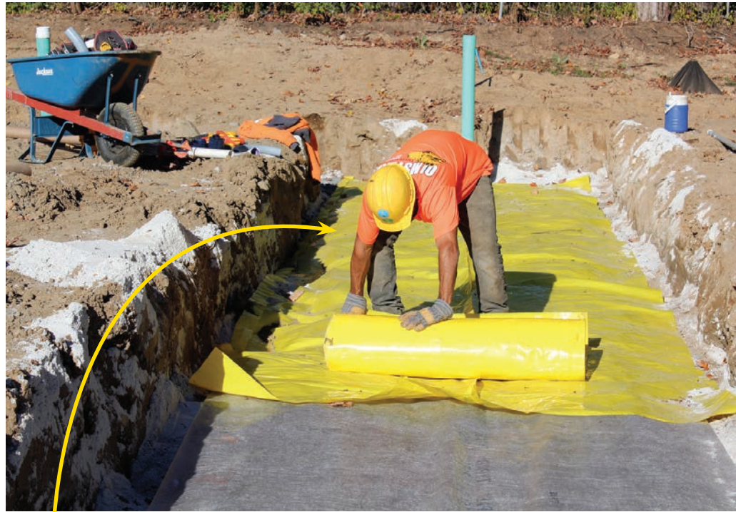
▲ Jose Vazquez from Olmstead Contracting lays 15-mil Stego Wrap vapor barrier over geotextile fabric to prevent air from escaping.
