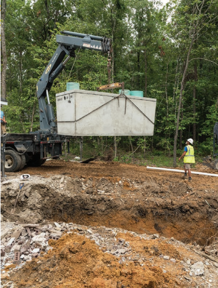
▲ Installer Joe Glover monitors an excavation site while Kevin Castleberry of Whitten Precast Concrete Products places a tank for a new onsite system.
