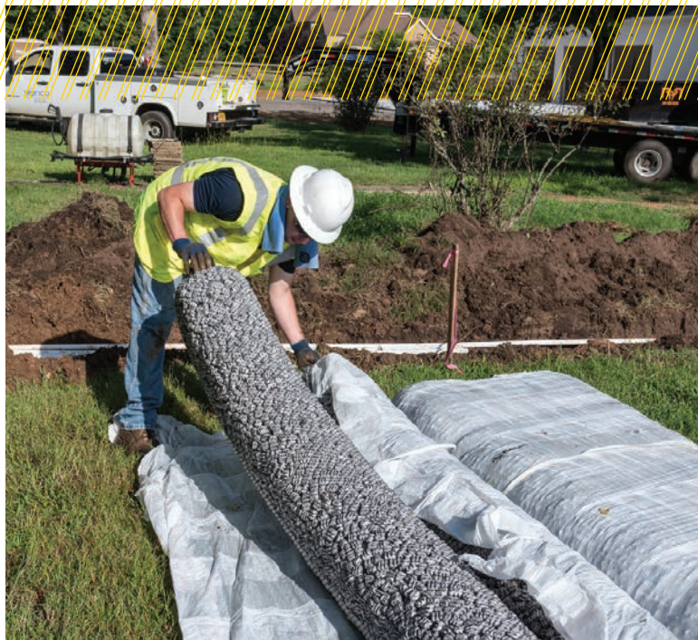
▲ Technician Adam Ault lays out an EZflow drainfield septic system from Infiltrator Water Technologies.
