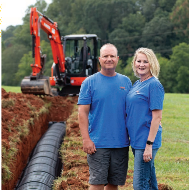
▲ Jarrid and Jeanie Lentz are shown at a work site where a Kubota excavator is digging trenches for a drainfield using Infiltrator Water Technologies chambers.
