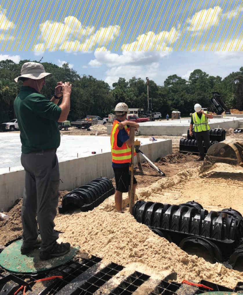
▲ From left, Chase Myers of Martin Septic Service photographs Woody Woodward and Greg Harris of Infiltrator Water Technologies preparing an excavated area of a drainfield installation on a Habitat for Humanity build site.
