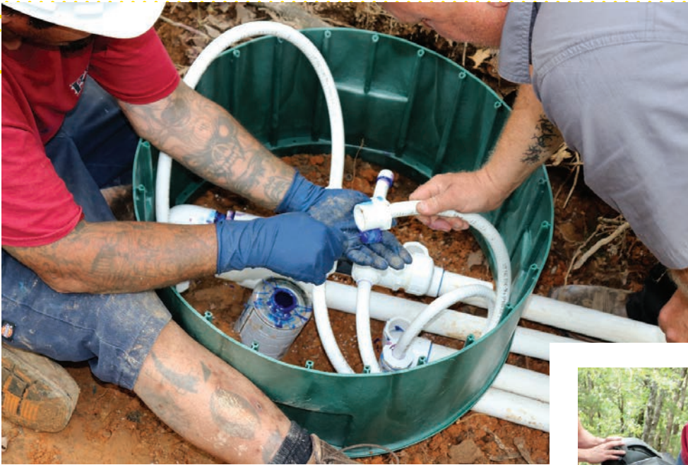
◀ Craig Mummert, left, and Brook Cannedy, senior installer for BBB Septic, hook up the Clarus Environmental spider valve assembly, enclosed by a 24-inch Polylok riser and lid.
