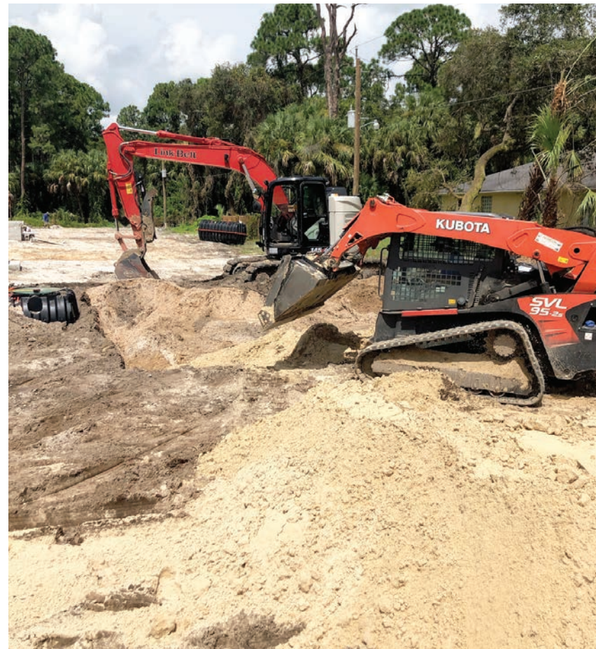
▲ Daniel Romer is at the controls of a Kubota skid-steer, covering a drainfield at the Habitat for Humanity site. Martin Septic Service has volunteered at Habitat home projects for 15 years.
