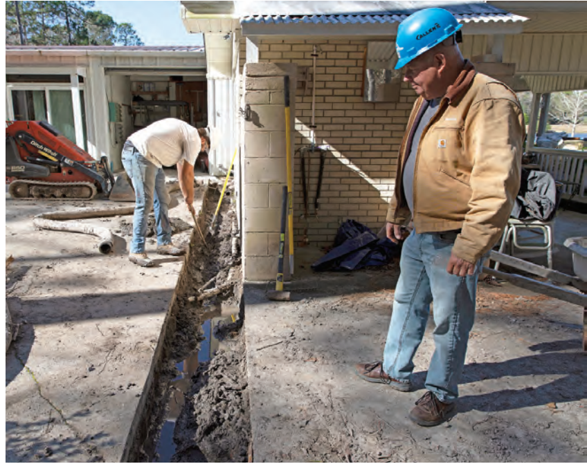
✔ Allen checks out the progress during an installation job. Josh Good works in the background.
