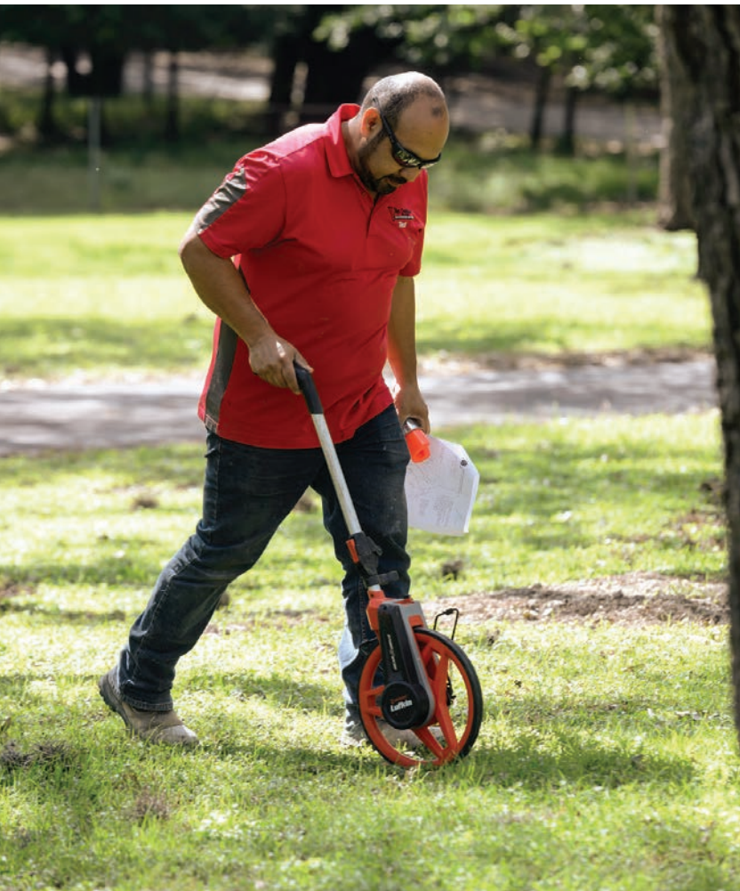
▼ Ted Talavara uses a Lufkin measuring wheel to mark trench lines during an installation.
