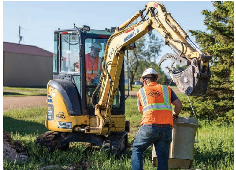
▲ These workers are wearing proper reflective vests and hard hats while moving components during an installation. (file photo)
