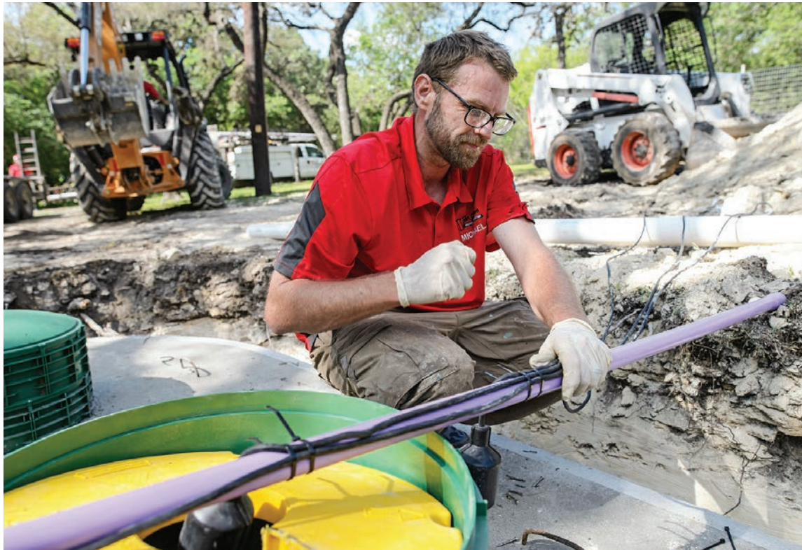
▲ Michael Foley works on electronic components while installing a residential septic system. Van Delden Wastewater Systems installs about 80 systems annually from Clearstream Wastewater Systems.
