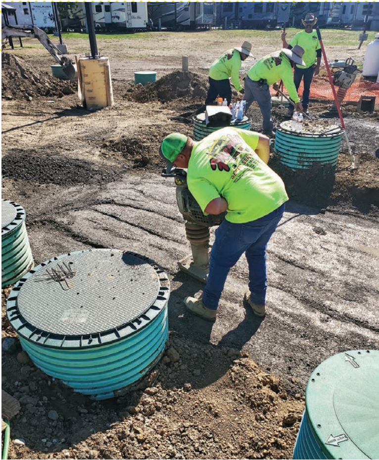
▲ The 2-inch force main from tank No. 1 to tank No. 2 followed the contour lines at the bottom of the hill.
