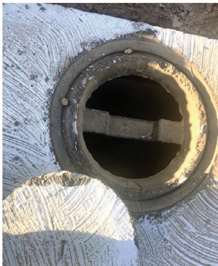
This contractor-submitted photo shows an inlet baffle that is located too close to the inlet pipe, which could lead to plugging with solids or toilet paper, as well as a customer call to the pumper for emergency service.
