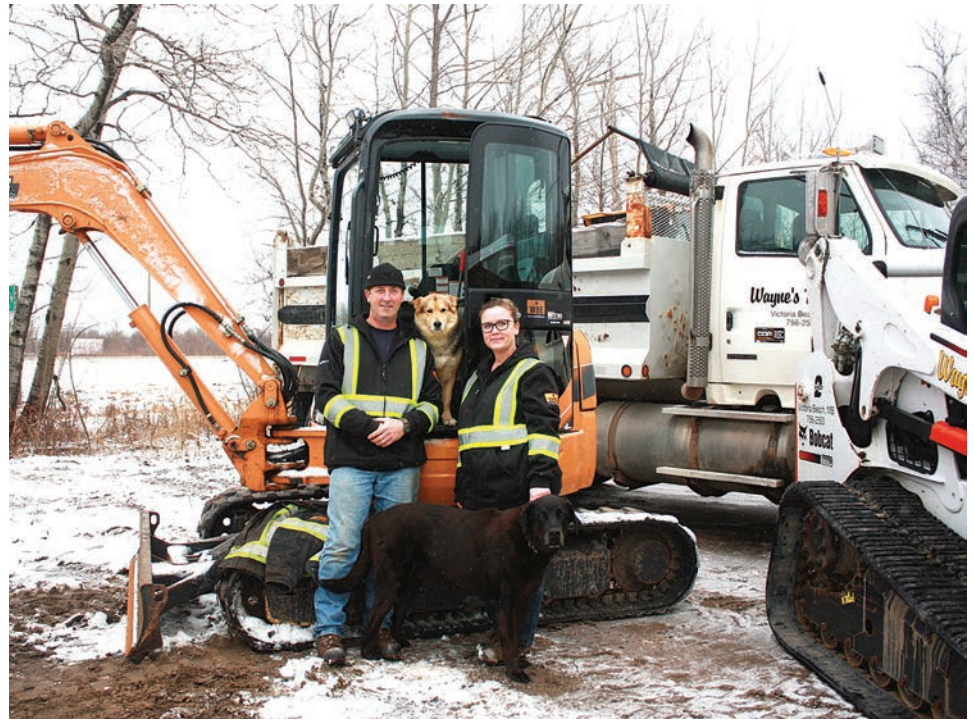
▲ Randy and Onale Thomas with Blue (in front) and Maggie (in the cab), a Case CX50 excavator, a 2002 Sterling tandem-axle truck with RENN dump box, and a Bobcat T770 compact track loader.
