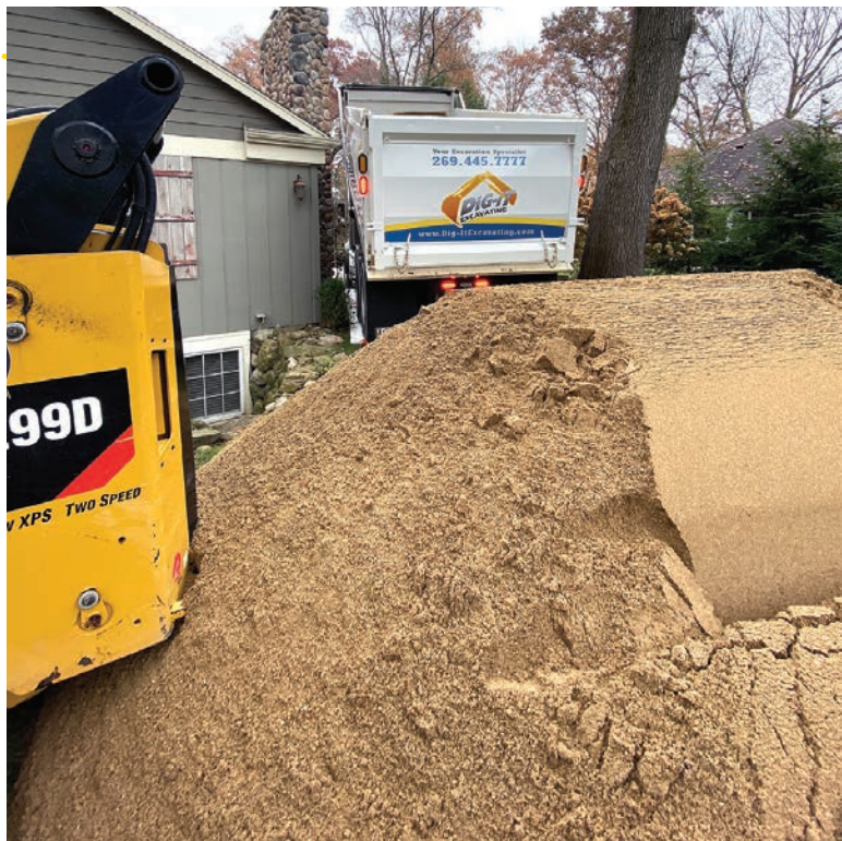
▲ There was little room to maneuver at the Dig-It Excavating job in northern Indiana. The Kenworth T880 was eased in next to the house to drop loads of fill sand, and the Caterpillar 299 track loader distributed it.
