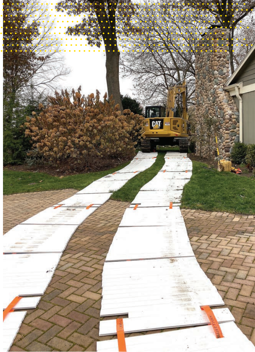
▲ A SlatTrax system of recycled plastic panels protected the driveway from damage at the Indiana project and also minimized compaction of the lawn when equipment was moved to the backyard job site, also when a big Kenworth T880 brought in loads of sand and fill.
