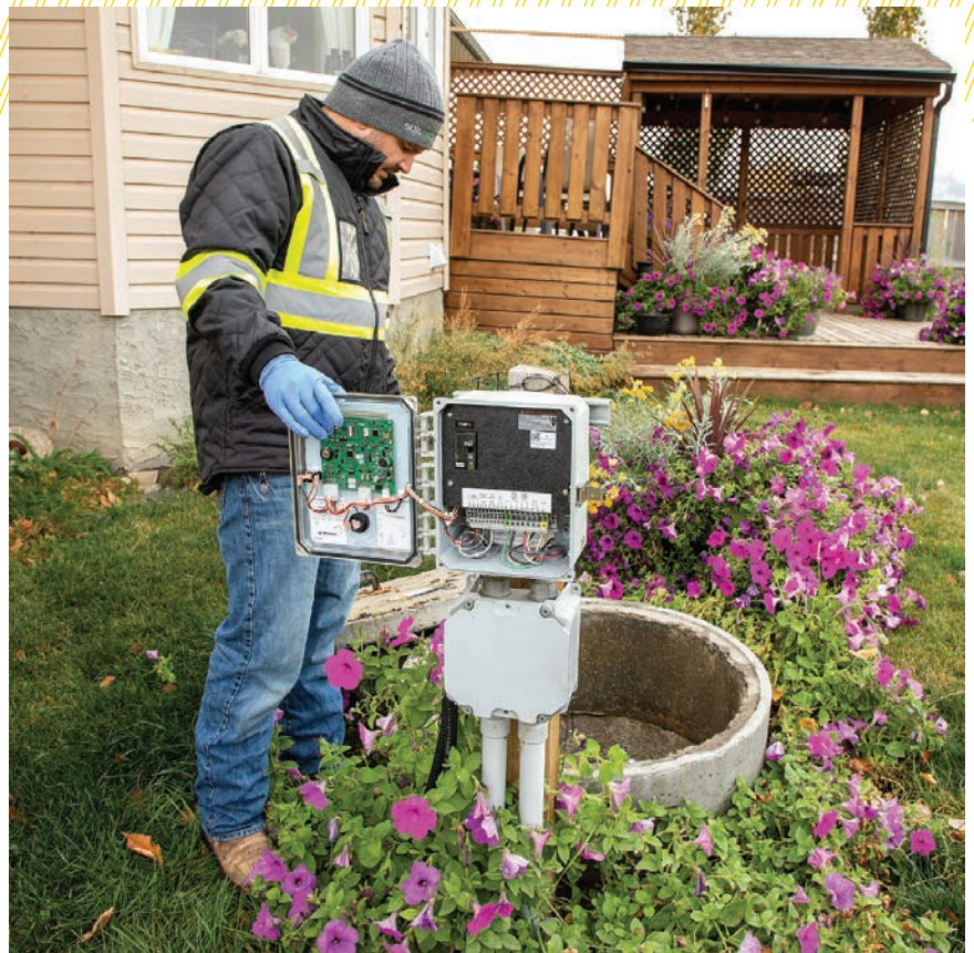
▲ Widmer activates the pump using a test button on the SJE Rhombus control panel during a septic system inspection.
