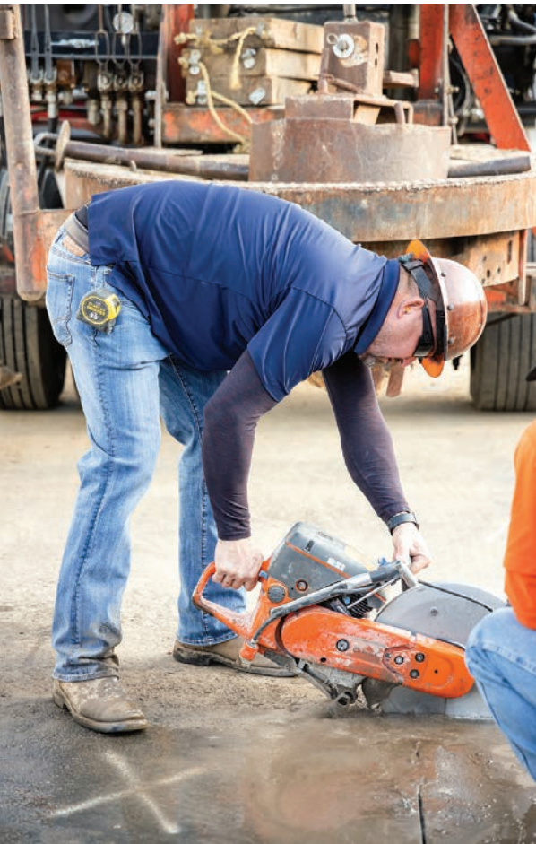
▲ Gilbert Herrera uses a Husqvarna K770 concrete saw to cut through asphalt to drill a test pit for a septic system for a commercial customer.
