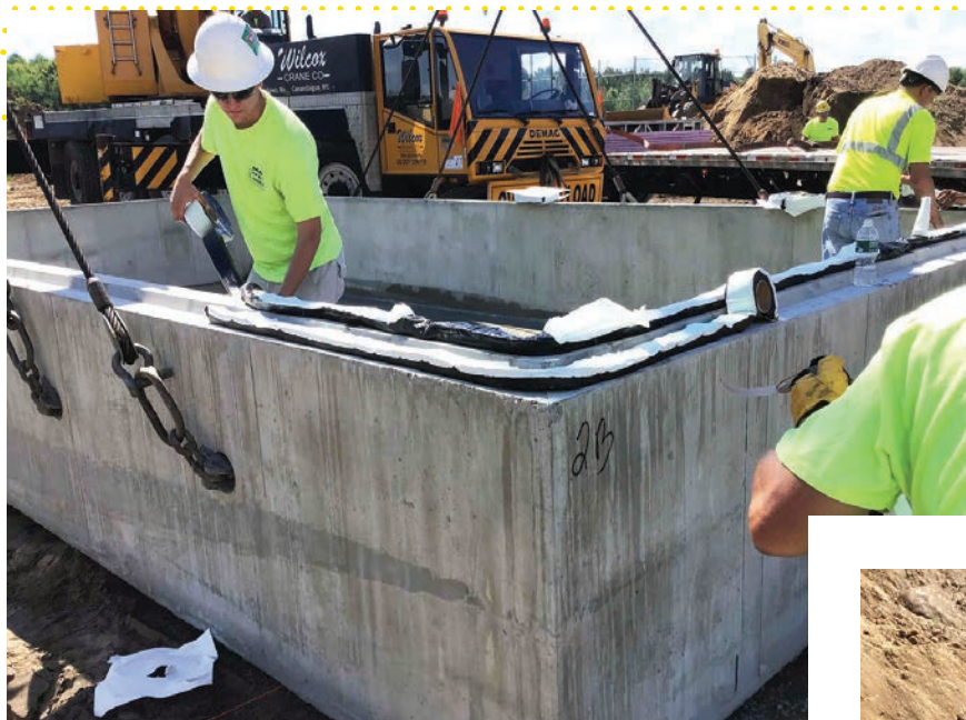
◀ Thomas Fiacco III (left) and Peter Arcadi from TJ Fiacco Construction apply butyl rope sealant to the bottom half of Tank 5. Barry Cook is in the background.
