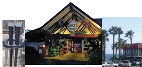
DUKE'S OCEANFRONT RESTAURANT, Malibu, CA 4 UV Unit Array Effluent Discharges into Ocean Beach Sand
