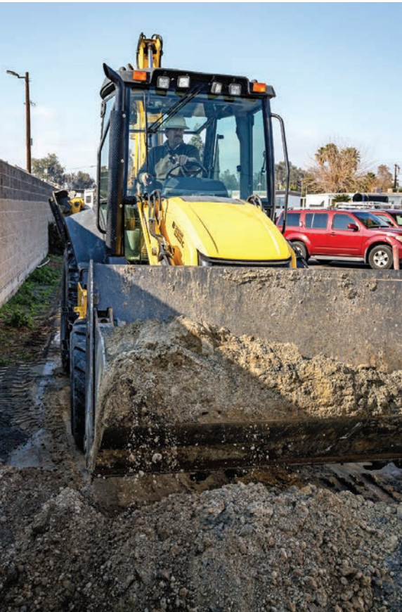
▲ Greg Shields uses a New Holland B95 backhoe to move excavated soil on a job site. (Photos by Matt Dayka)
