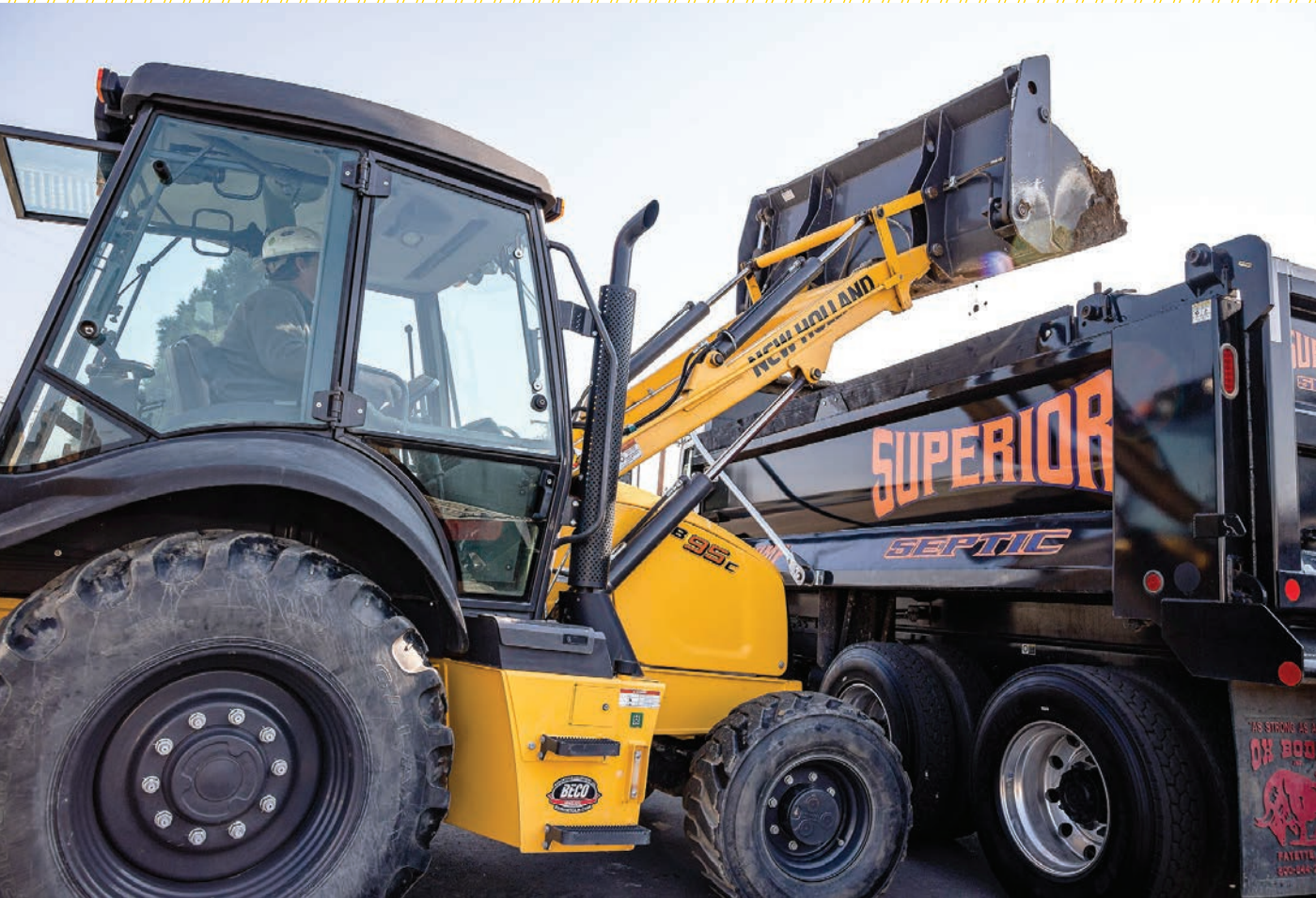
«Greg Shields uses a New Holland B95 backhoe to load spoils from a test pit into a 2020 Peterbilt 10-wheel truck with an Ox Bodies dump body.
