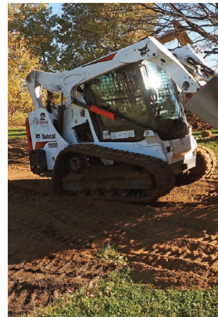
▼ Joe Rubenzer uses a Bobcat compact track loader to move topsoil during the construction of a mound system.
