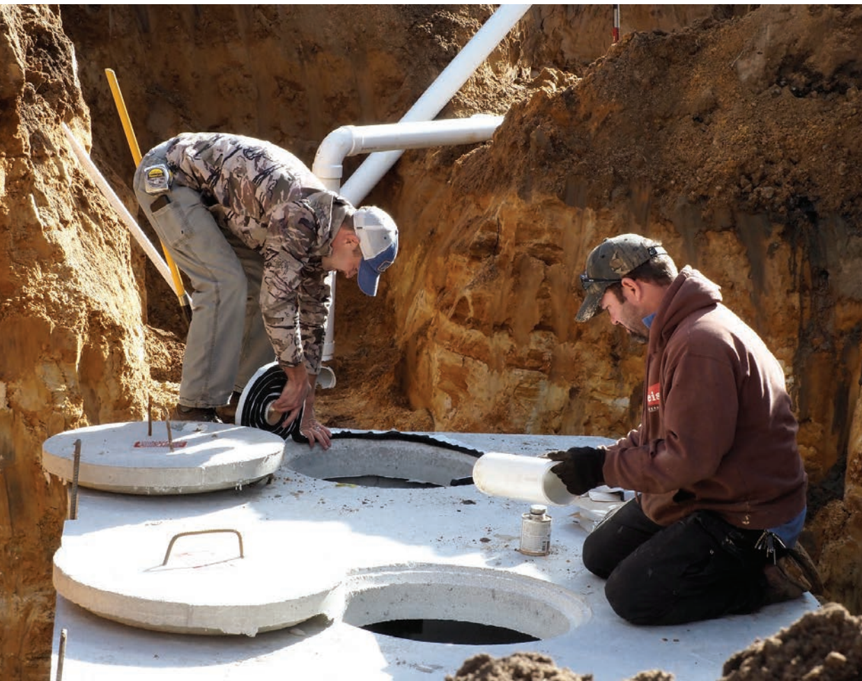
◀◀ Joe Rubenzer, left, and Mark Yohnk prepare a concrete tank from Skaw Pre-Cast for concrete risers.
