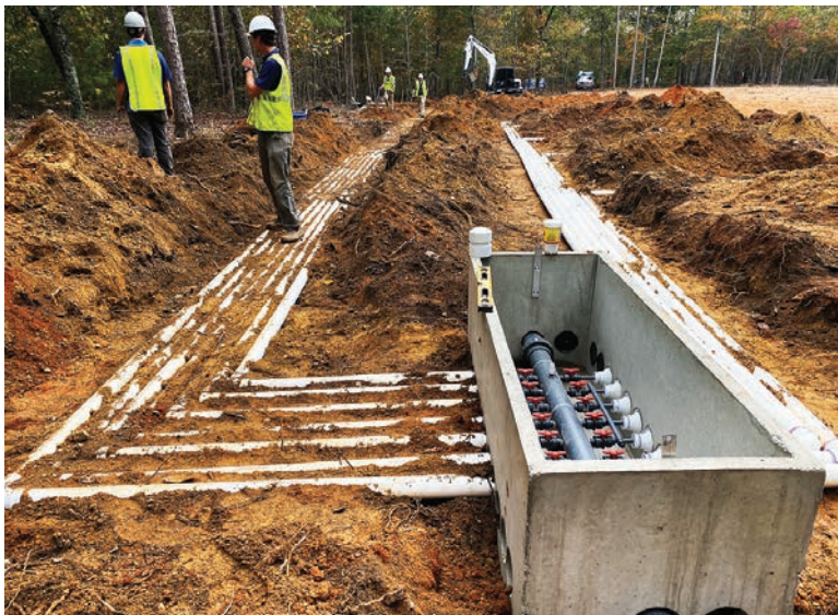
▲ A 14-tap manifold with supply lines.
