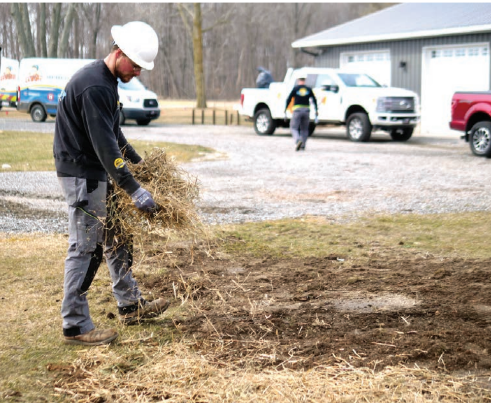
« James Sanders spreads grass seed and straw after repairing a residential sewer line.
