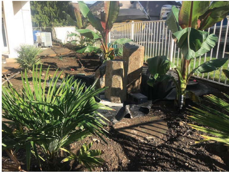
▲ The Lake Tapps property was large, but the house consumed most of the width. Technicians had only a few feet to work with and had to stage construction because there was no extra space for piling dirt. The rocks in the foreground are artificial and conceal the tank lids.
