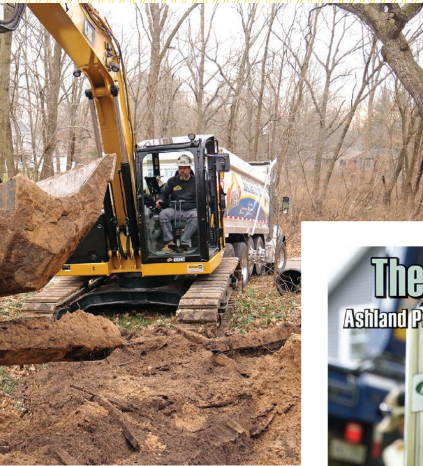
◀ Dervin Witmer operates a Cat 310 excavator equipped with an Engcon tiltrotator as he clears brush to install a riser to an onsite system.
