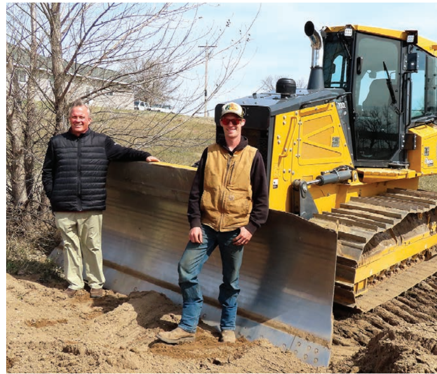
▲ Vern Schnathorst, left, the work-based learning coordinator for Detroit Lakes High School in Minnesota, and student Jaden Thorson are shown on a work site with a John Deere 700L crawler dozer. (Photos provided by Vern Schnathorst)
