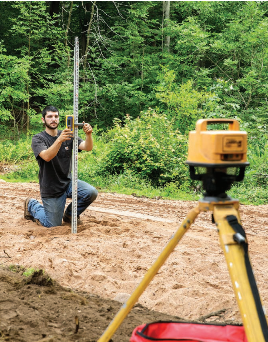
▲ Mike Camarota uses a Spectra Precision LL500 laser level to determine the grade for a distribution box installation. (Photos by John Marinelli)
