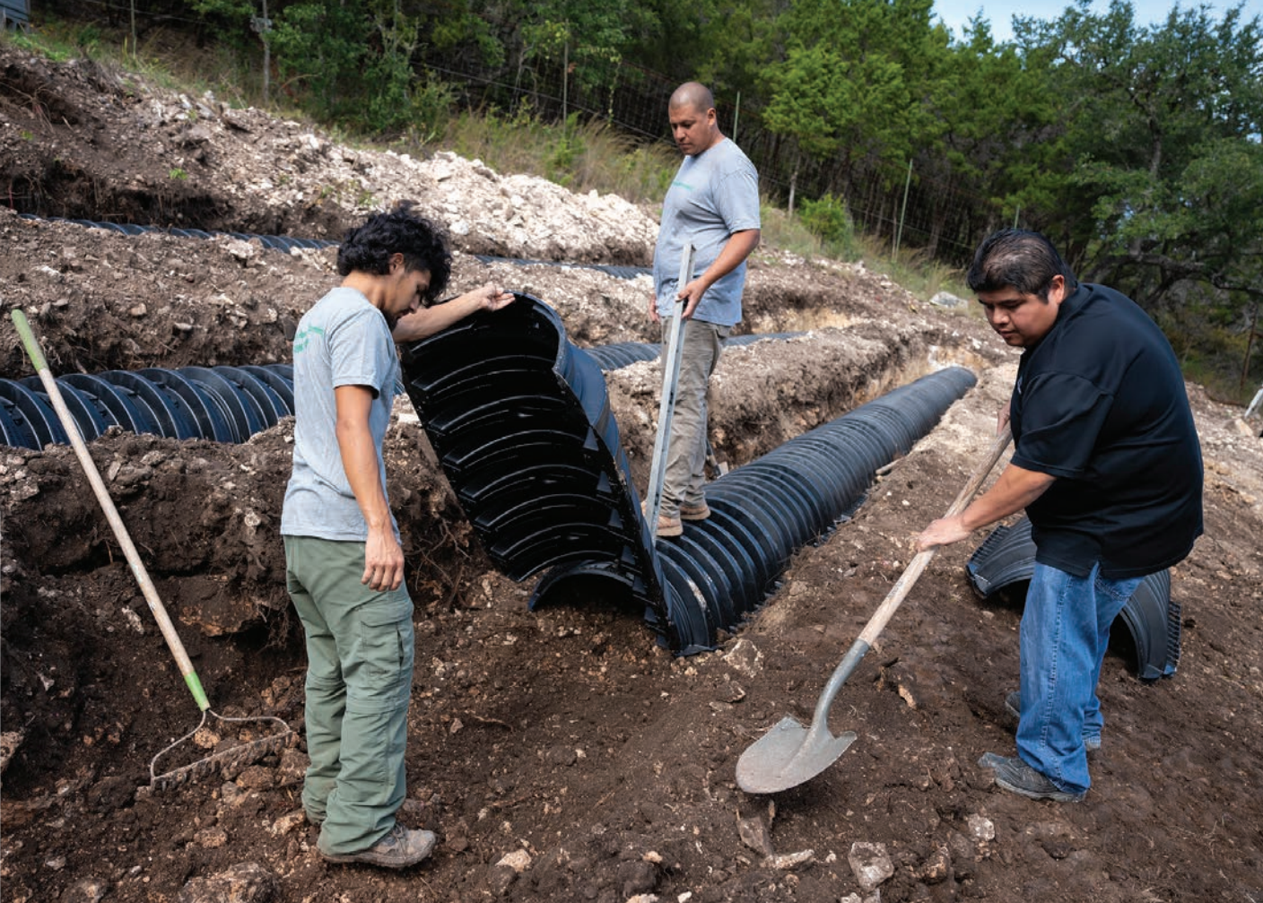
◀ Orlando Godinez, right, works with technician Alex Aguilar-Murillo, left, and lead technician John Ibarra, background, to install chambers from Infiltrator Water Technologies.
