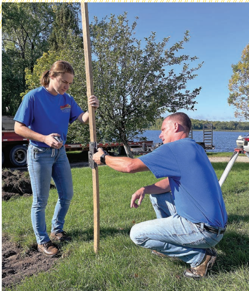
▲ The Ohms use a Nikon AL-15 laser level during a septic system installation.
