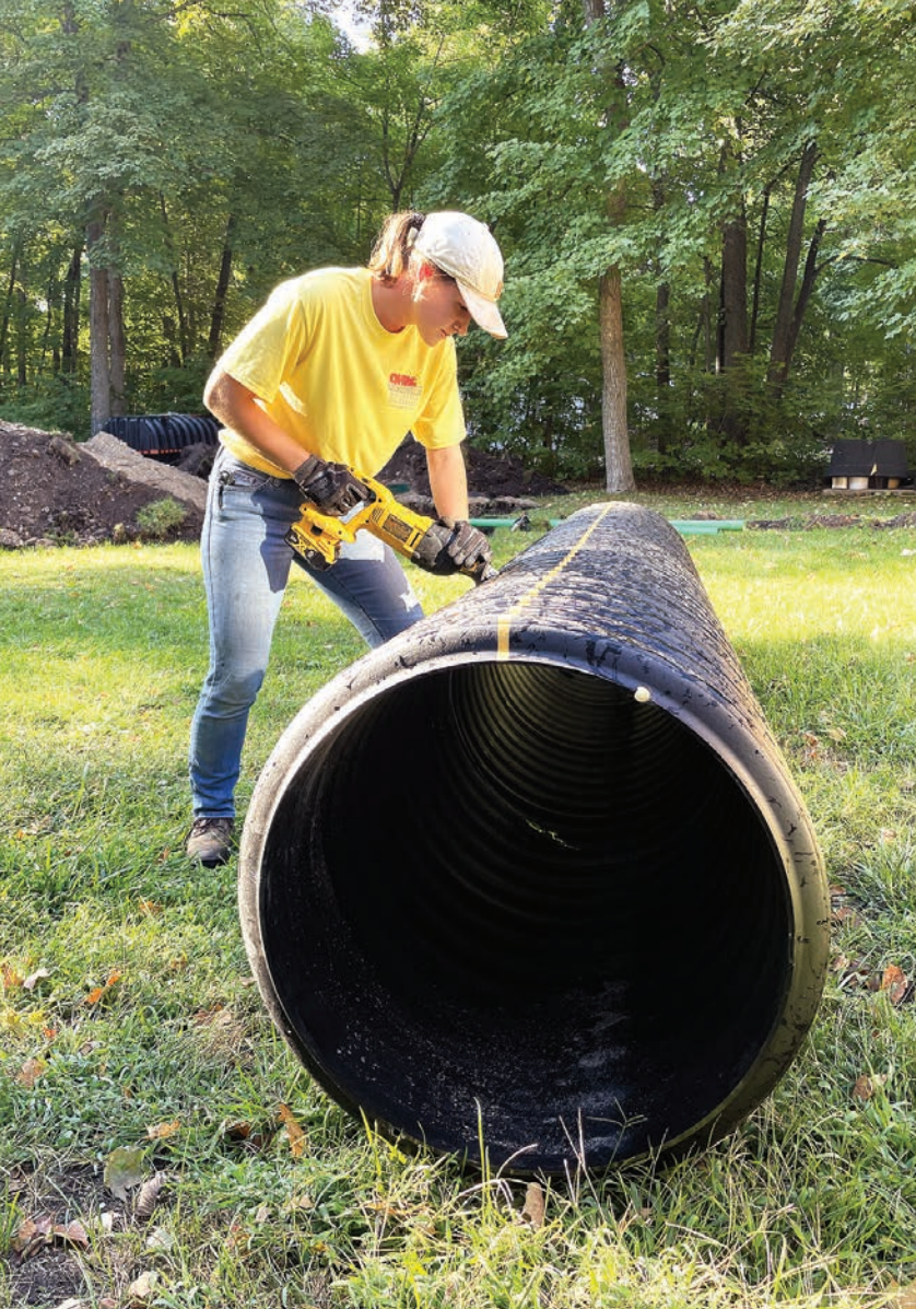
◀ Olivia Ohm cuts a length of plastic pipe on a job site.
