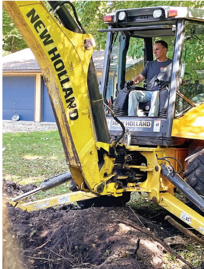
▼ Chris Ohm is behind the controls of a New Holland backhoe during an installation.
