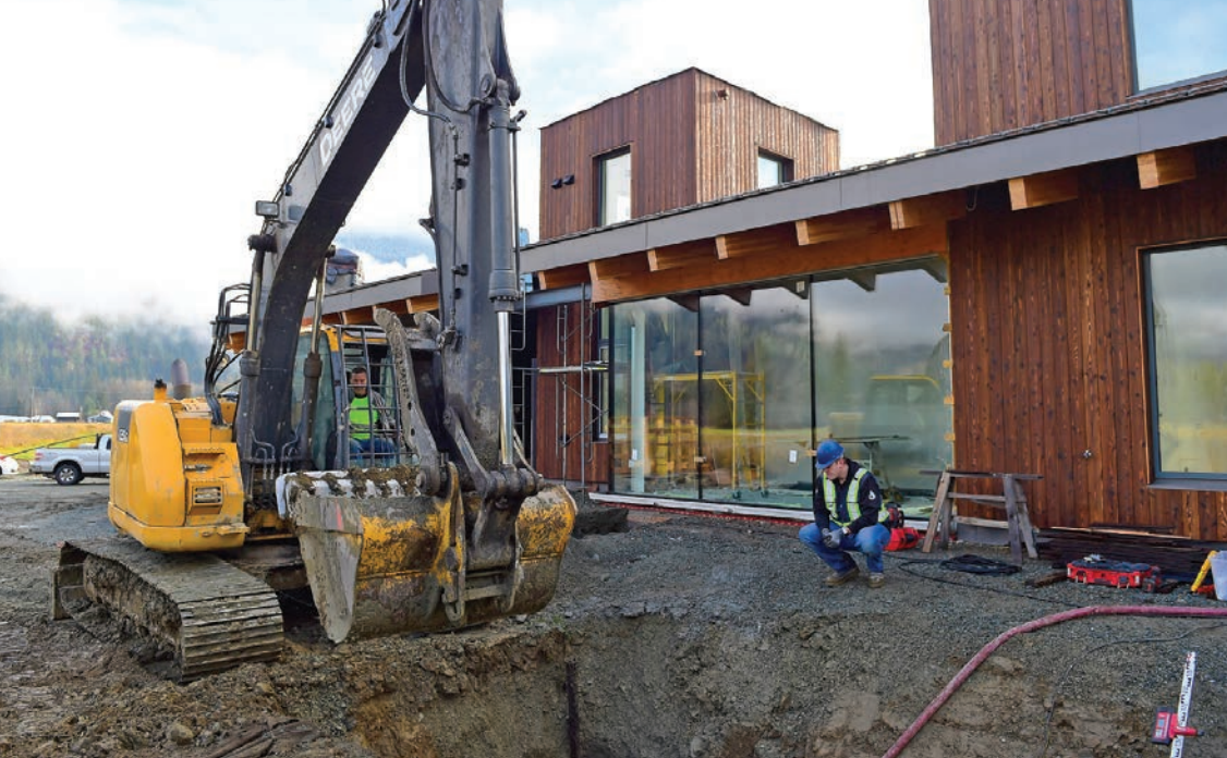
◀ James Stiksma supervisors a subcontractor operating a John Deere excavator on a residential system installation in Pemberton, British Columbia.
