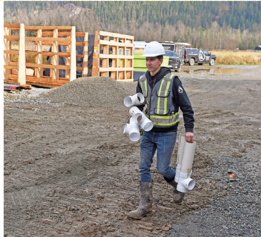
▲ Brouwer carries PVC pipe fittings during an installation project for a new home.
