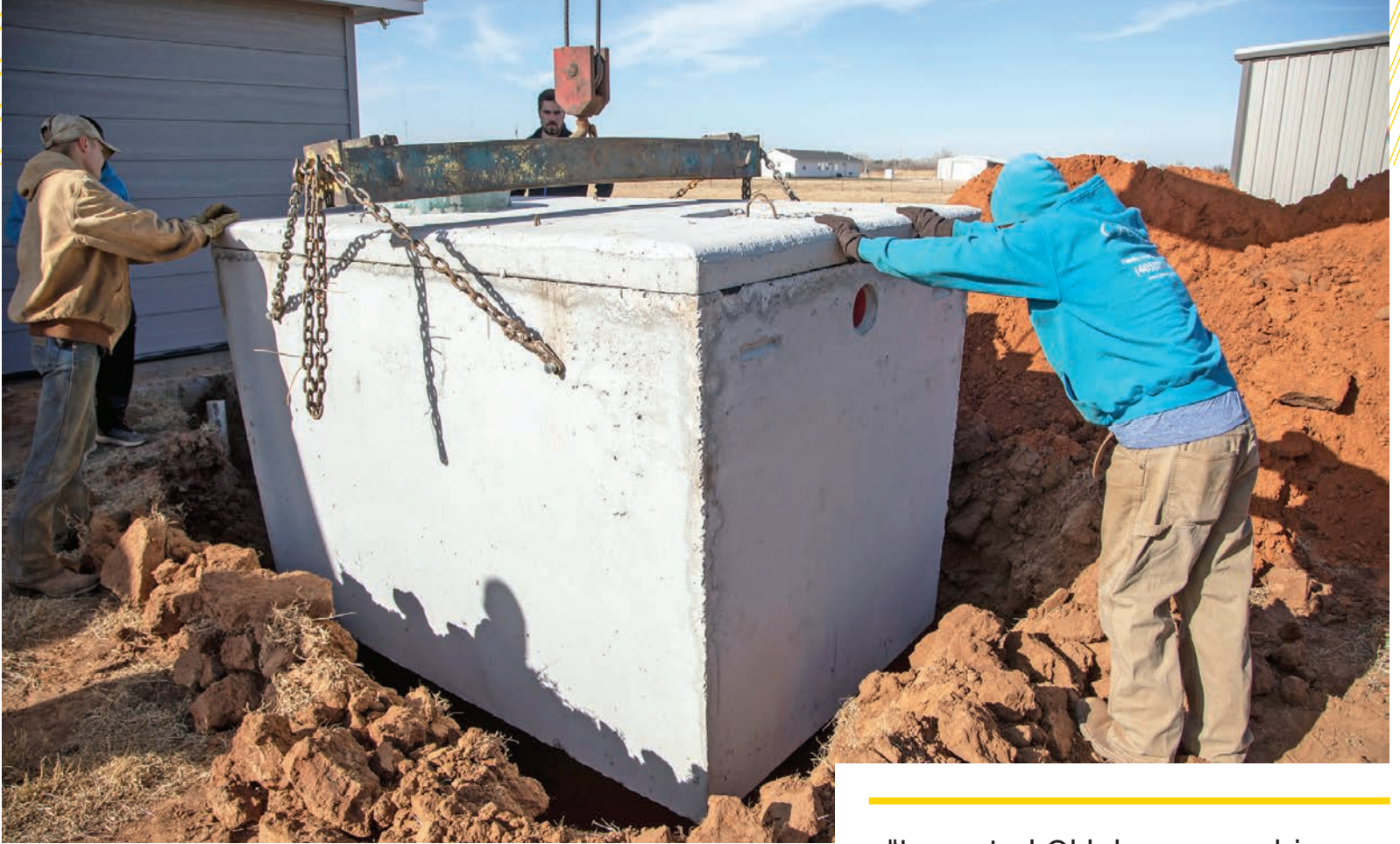
▲ Levi Karcher helps guide a septic tank into the ground at a residential work site.
