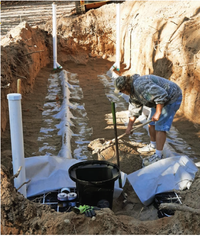
◀ Greg Golden distributes sand over the top of fabric protecting the Eljen GSF treatment modules. Observation vent pipes are shown in the background.
