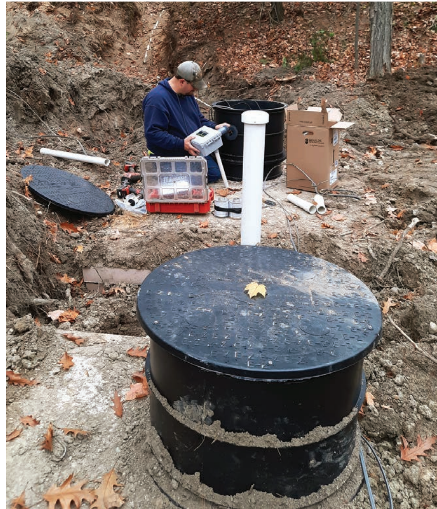
▲ Dustin Augustine installs a JB Plugger dual-float control from SJE Rhombus. The riser and lid are from Infiltrator Water Technologies.
