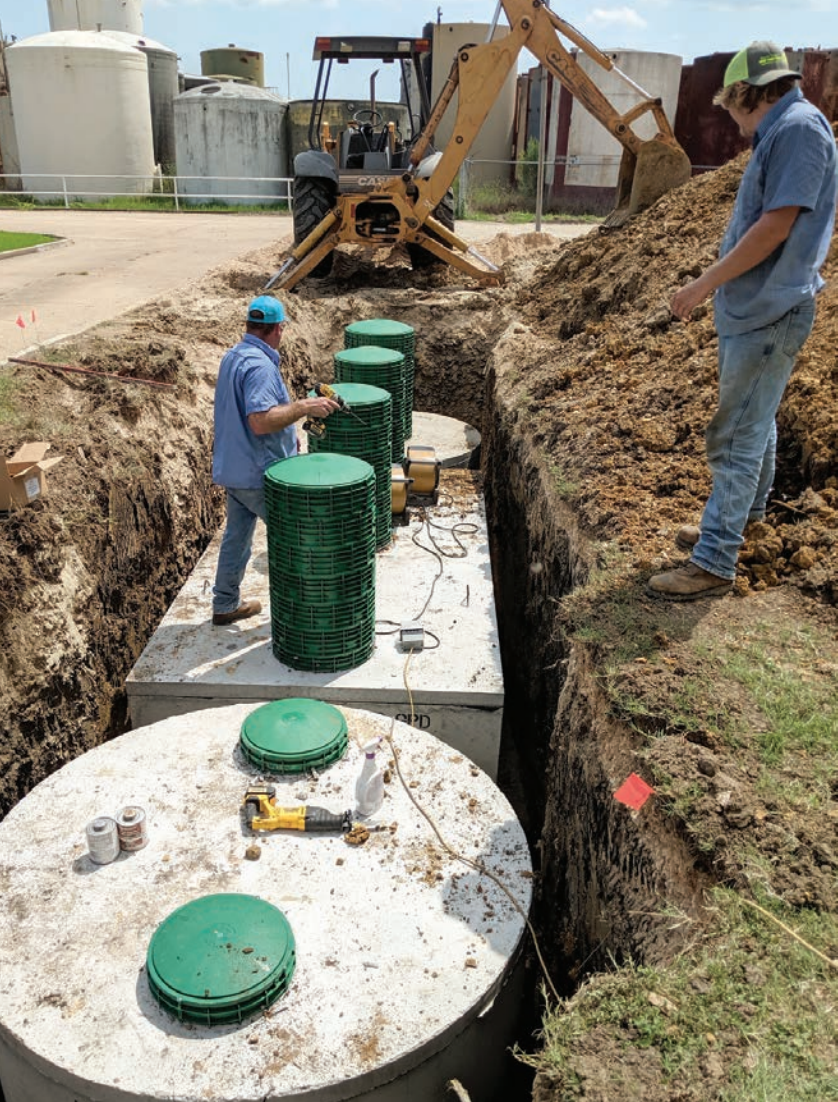
▲ Al installs a riser while Eric looks on. The tanks are part of a 1,500 gpd system installed at an oil field site.
