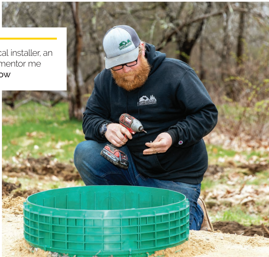
▲ Derek Boudreau works with a Tuf-Tite riser and lid on a new septic tank installation.
