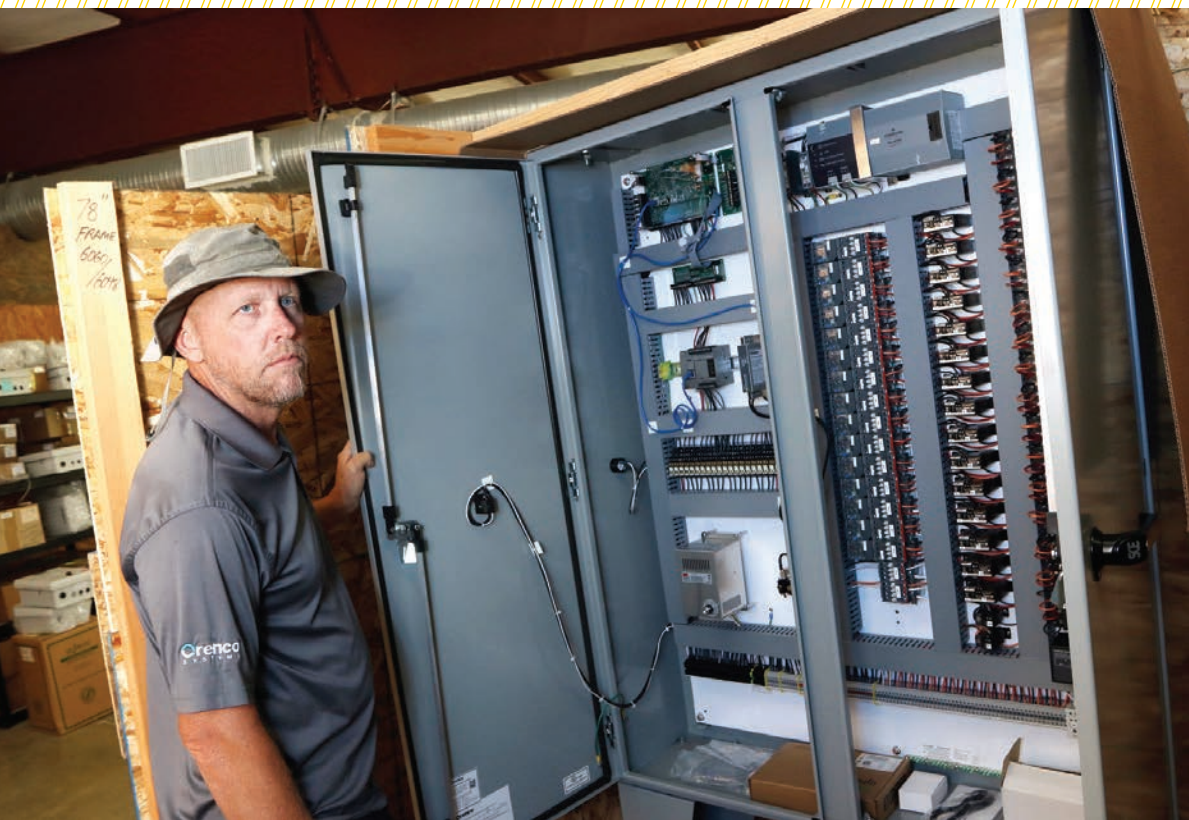
◀ Steve Barry looks over a TCOM custom control panel set to be installed as part of an Orenco commercial wastewater treatment system.
