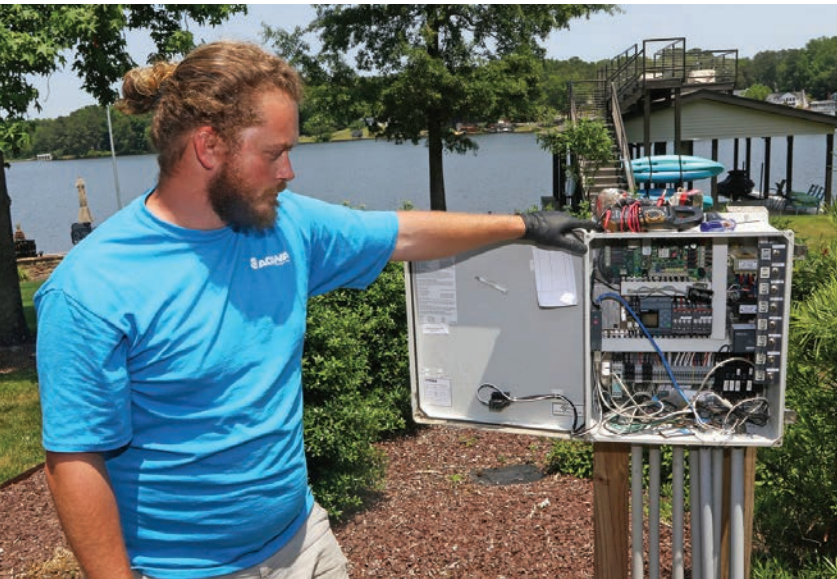
◀◀ Jonathan Handley checks a VeriComm control panel that is part of a new Orenco AdvanTex system installed during a residential project.
