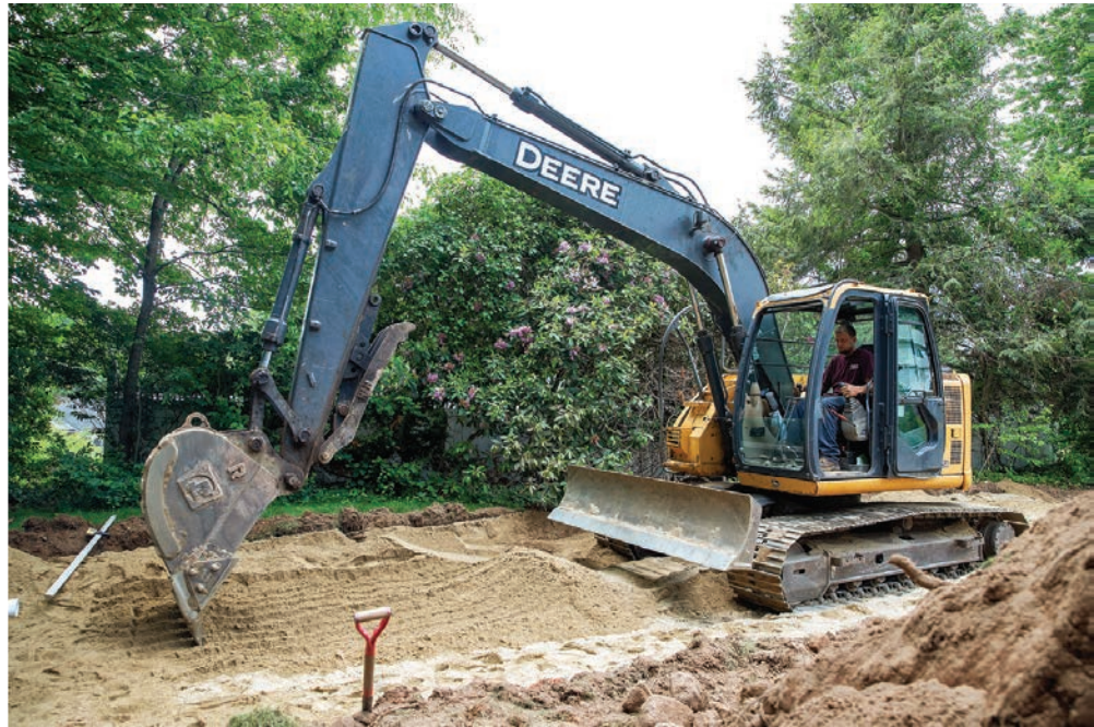
▲ Josh Gondek is at the controls of a Deere excavator during a septic system installation for County Line Septic.
