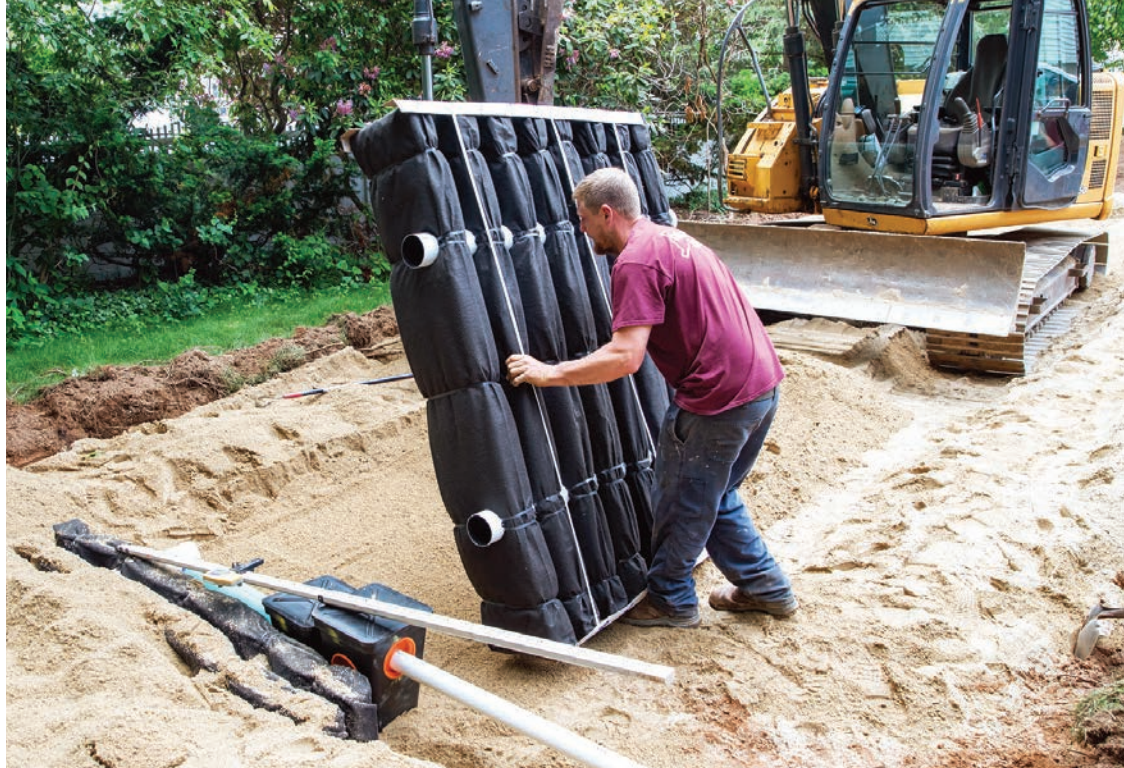
➤ Josh Gondek places a Mantis unit from Eljen into a drainfield for a new septic system.
