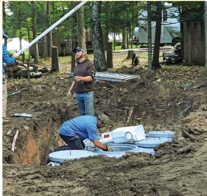
▲ Forest Clement (standing) and Mark Yohnk from Stolt Excavating install the Polylok 525 effluent filter in the Huffcutt Concrete 1,000-/600-gallon combination tank.
