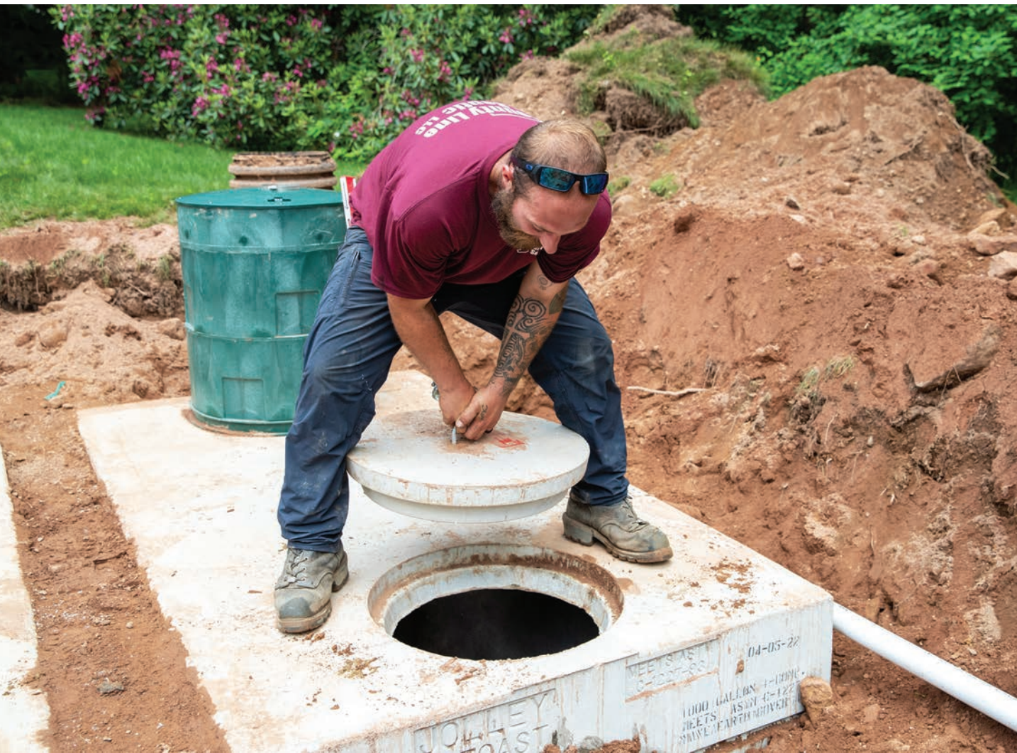
◀ Paul Meikle installs the cover on a concrete pump chamber while building a septic system.
