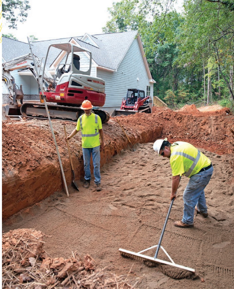
▲ During a system install, Harold Kilgore smooths sand in a trench as technician David Thompson looks on.
