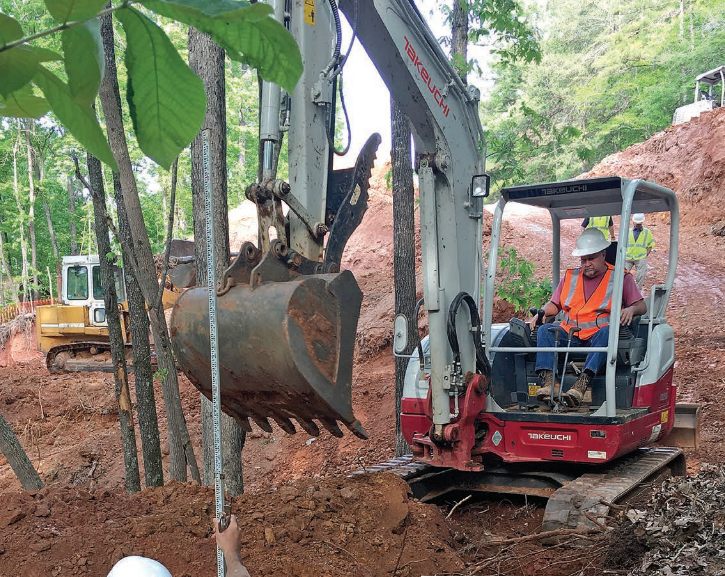
◀ Harold Kilgore is at the controls of a Takeuchi excavator during a challenging installation on a sloped property. (Photo courtesy of Harold Kilgore)
