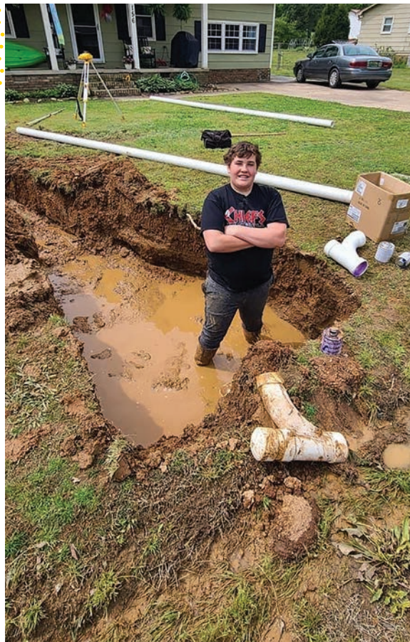
▲ In the trench shooting grades is one of C.J. Gulley's favorite places to be at an installation work site.
