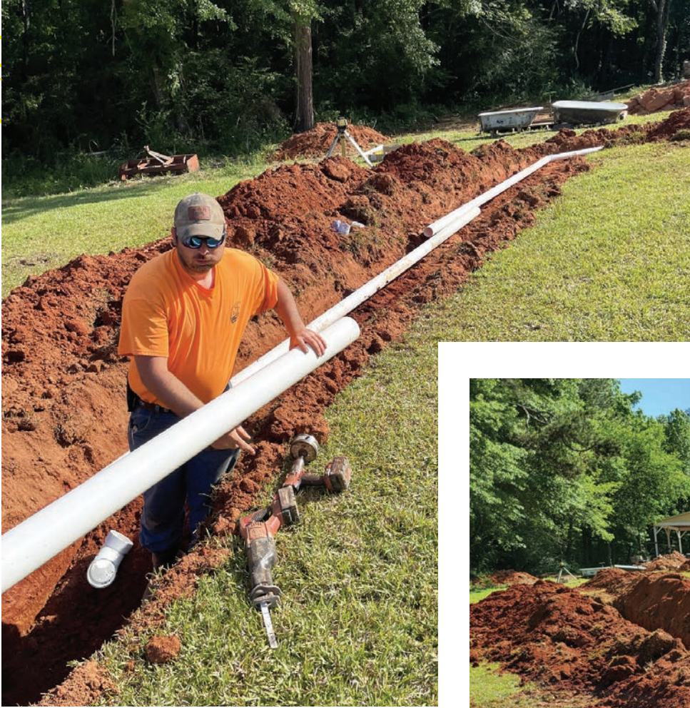
◀ A technician formerly with Geiger's Septic Services lays the PVC pipe from the septic tanks to the dispersal field.
