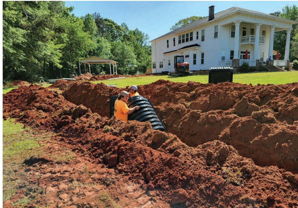
▼ Andrew Pugh (left) and Chris Sims, technicians from Geiger Septic Services, installing the Infiltrator Quick4 Plus chambers with the Exodus Ranch home and Kubota excavator in the background.
