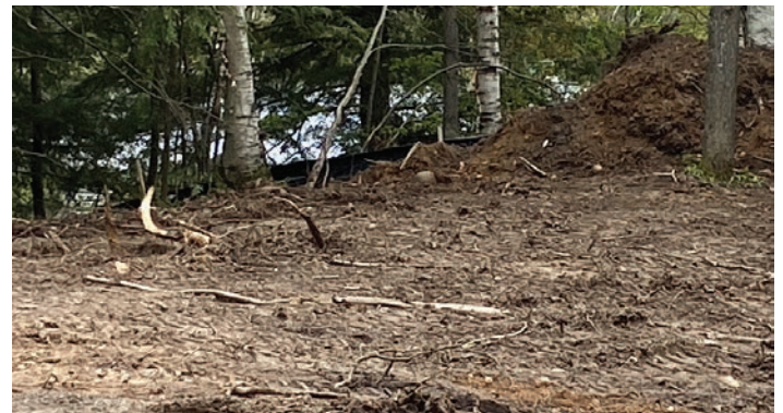
⚠️ The silt fence is not likely to contain the disturbed soil on this work site. (Photos courtesy of Jim Anderson)
