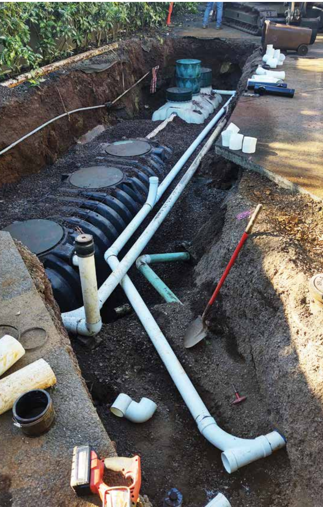
▲ Mike Cowper and Kris Magaellous worked for two weeks to hammer out this 20-by-8-by-10-foot-deep excavation. The pretreatment tank with three White Knight Microbial Inoculator Generators (Knight Treatment Systems) is in front of the Fuji Clean USA aerobic treatment unit. (Photos courtesy of Mark Noga)
