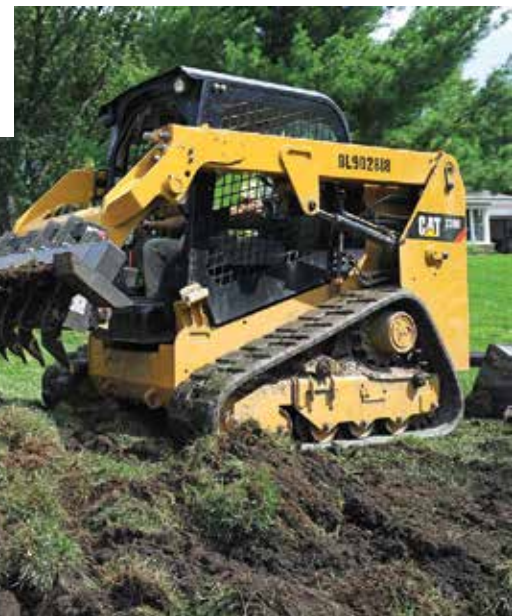
▼ Bishop uses a chisel plow attachment on a Caterpillar skid-steer to create the base of a modified mound for a replacement system.
