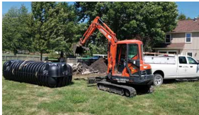
▼ A Roth North America plastic septic tank is installed using a Kubota KX121-3 mini excavator.
