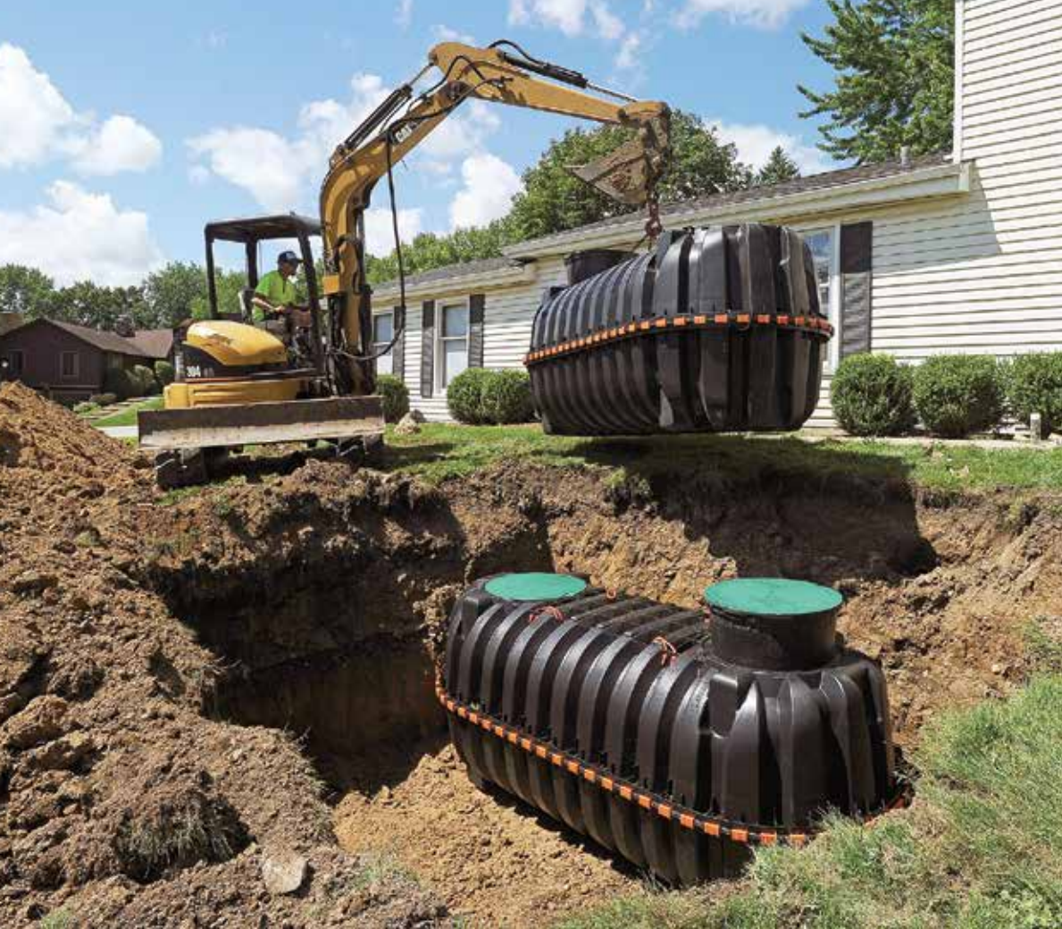
◀ Johnson is at the controls of a Caterpillar excavator, placing a pair of tanks from Infiltrator Water Technologies.
