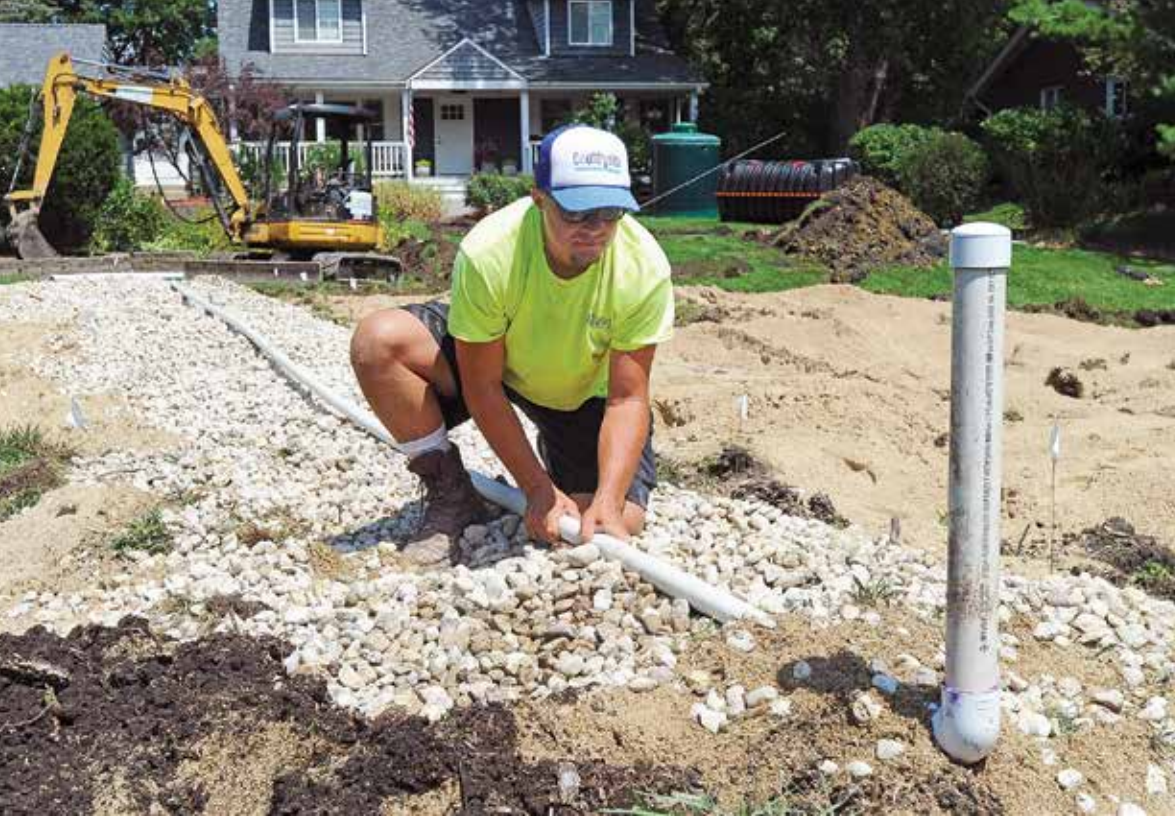
◀ Johnson lays a pipe and inspection port for a mound system at a home in suburban Chicago.
