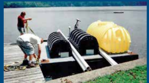
▲ Employees George Rosselli (left) and Chris Chernes prepare to lash the septic tank and chambers to the 12-by-12-foot powered wooden dock.
