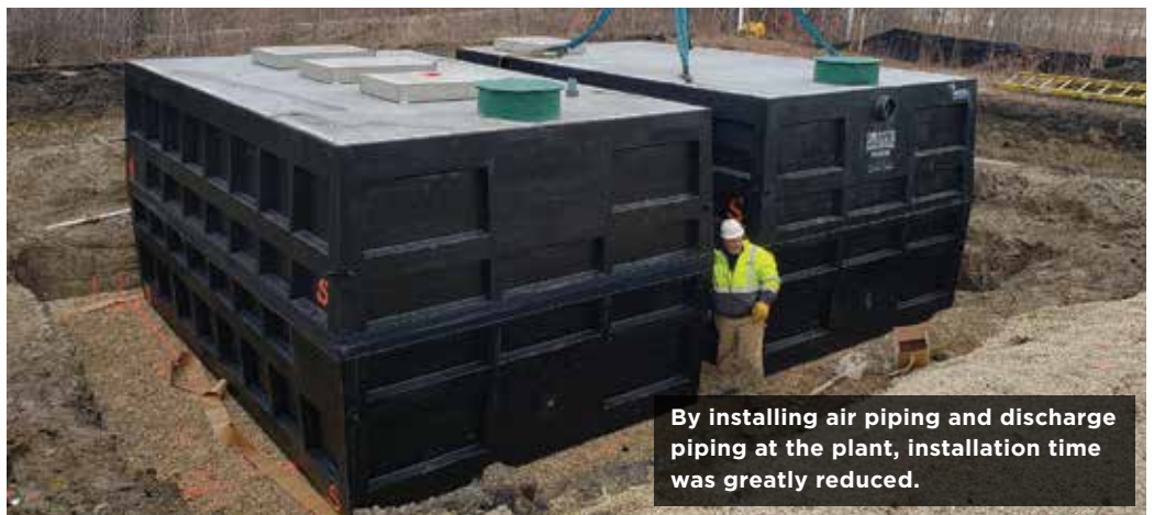
Workers install 12,000-gallon precast concrete tanks for a development in the Midwest.
