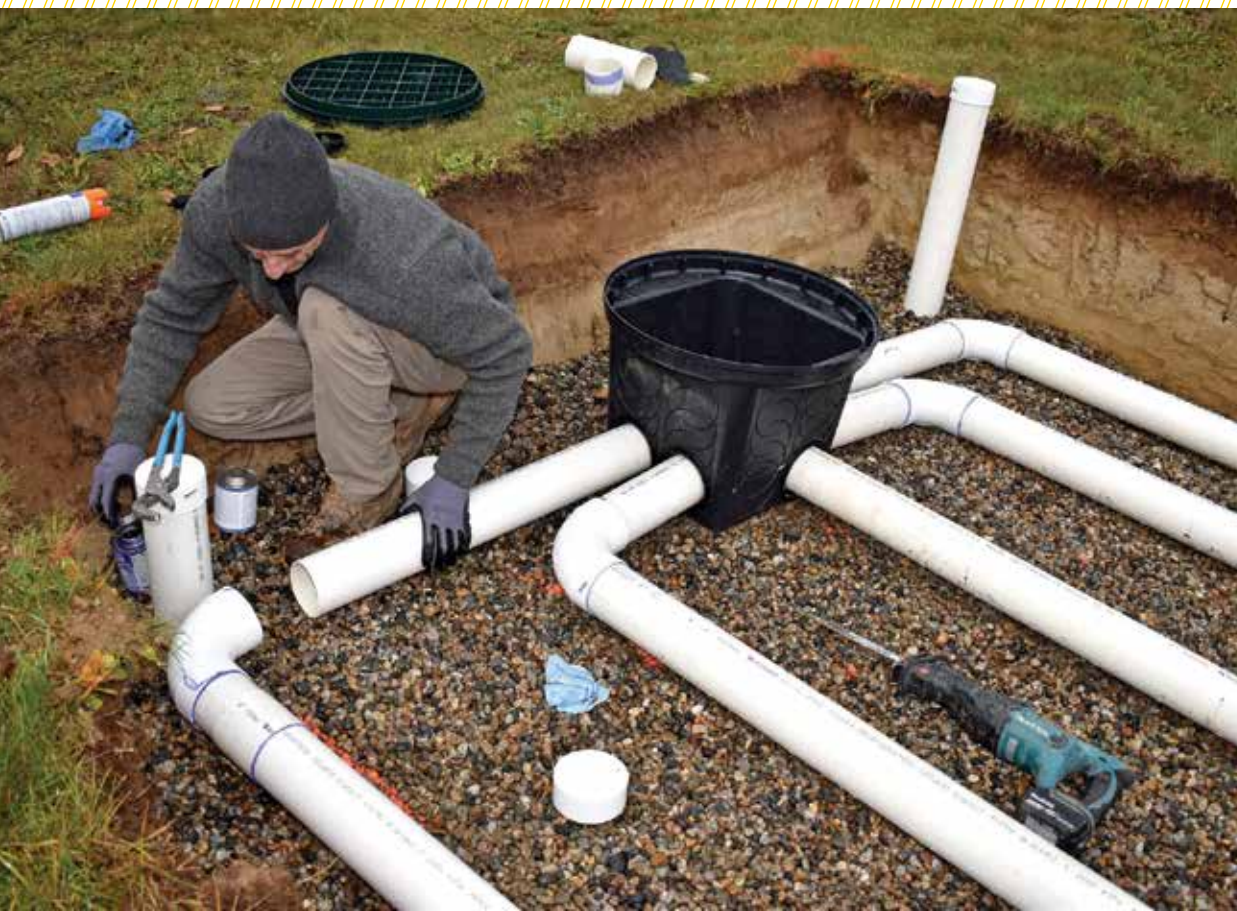
◀◀ Karthein links PVC drain pipe coming from a distribution box.
