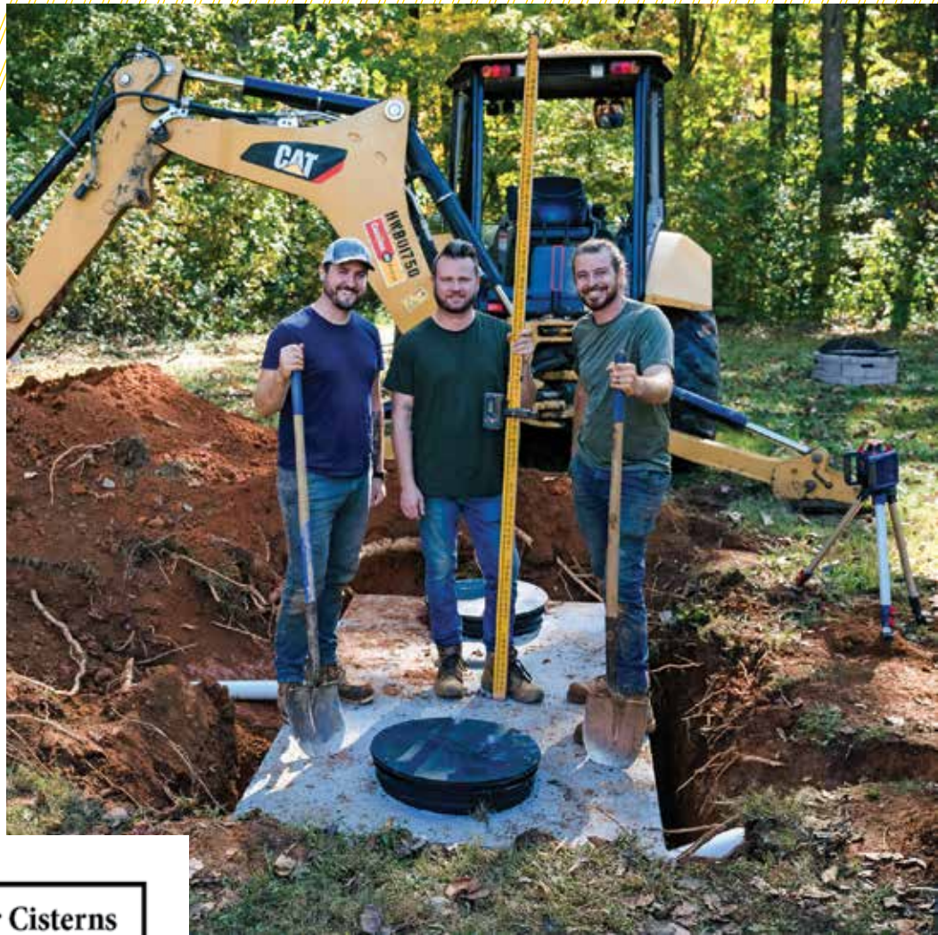
» The crew of John Paul McLaughlin, Matt Gravely and Shane Broyhill are shown during a septic tank replacement.
