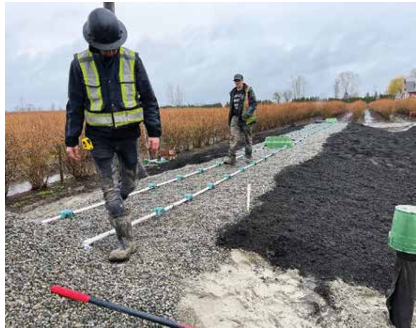
▼ Arien Brouwer of Canadian Septic, left, and a contractor's technician walk the top of the finished sand bed. Pipes are set on a 4-inch bed of 1/2-inch drain rock to aid water dispersal.
