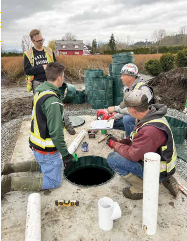
◀ Jim Smith of WestCoast Telebelts, top right, briefs the crew about the potential hazards of working around a Telebelt system at the project in Abbotsford, British Columbia.
