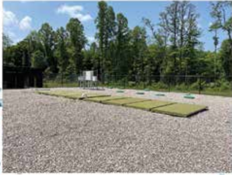
Elementary School, OH 6000 GPD
