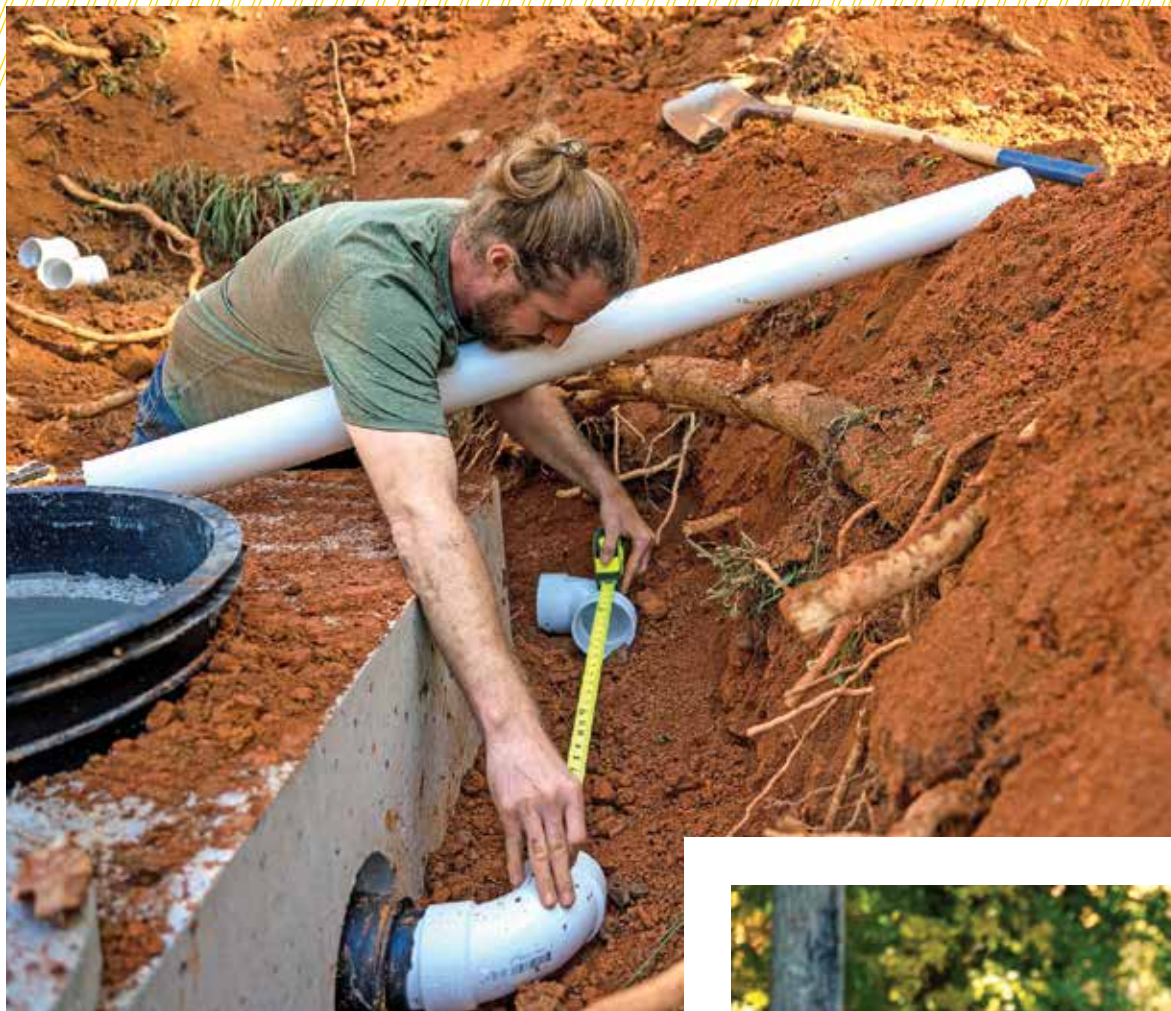
◀◀ Broyhill fits the outlet piping coming from a replacement septic tank on a residential onsite project.
