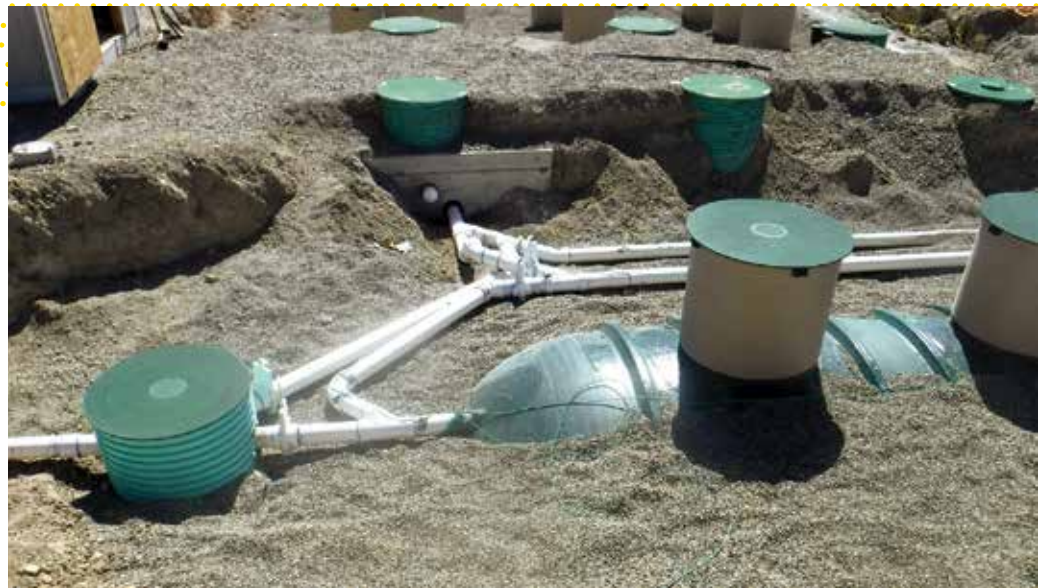
▲ The head end of the 13,000-gallon Xerxes tank shows the influent pipe and beyond the recirculation line and the influent line leading from the Xerxes tank to the first set of three 3,000-gallon tanks in the next stage of the treatment chain.
