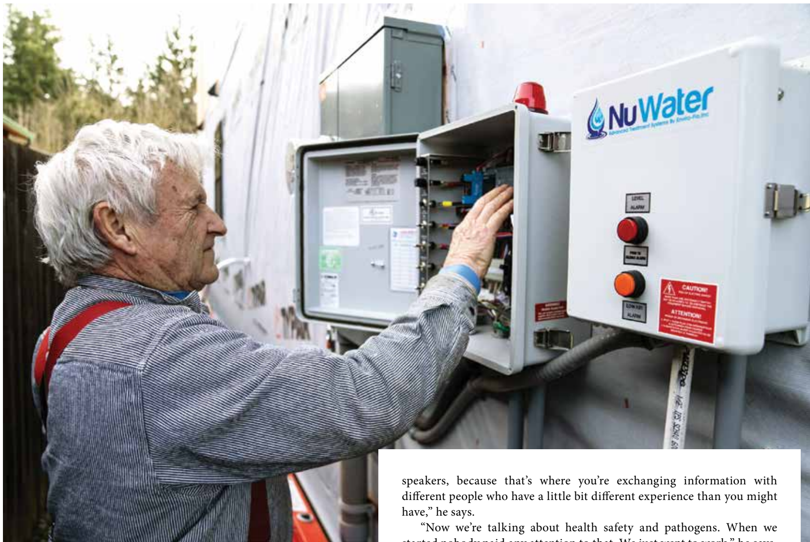
▲ Stonebridge checks an Orenco Systems control unit in a NuWater aerobic treatment unit in Clinton, Washington. Inspections make up about 20% of the company's workload.
